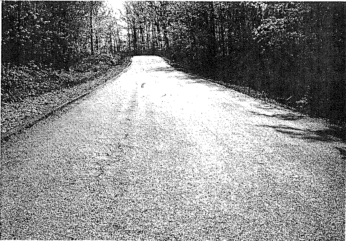
Fig. 11. Livingston County, SP70-730. Rutting and Cracking in Cut Section. The area in distress is approximately 100 feet long. (4-22-64)
