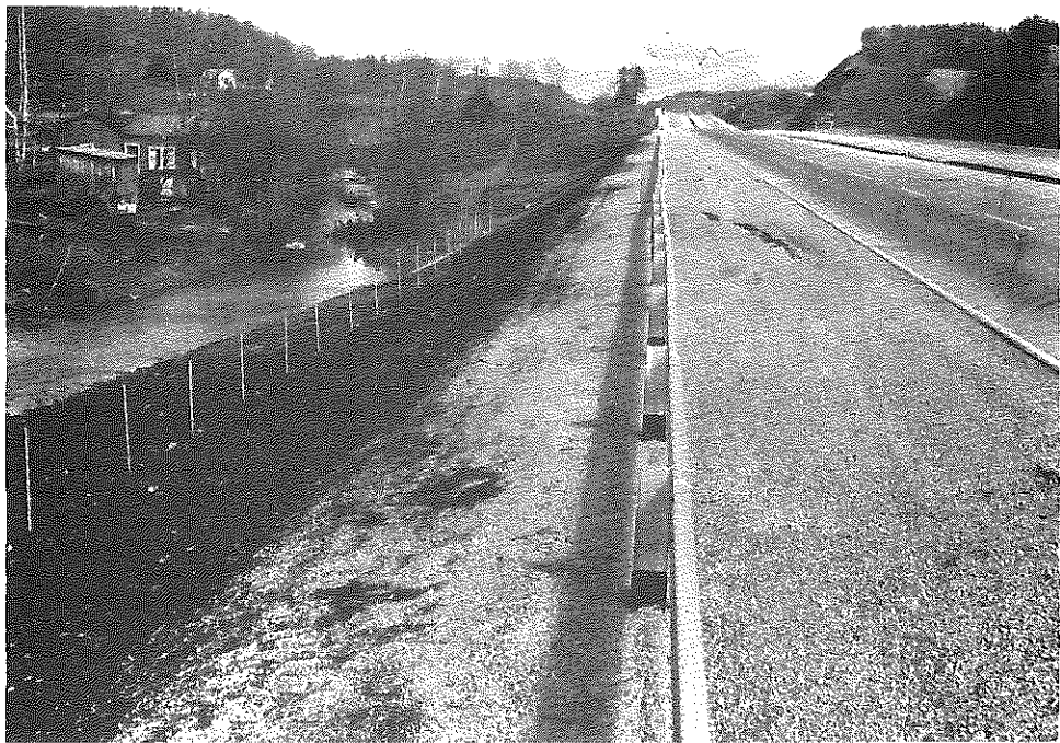
Figure 35. Landslide Area on the Mountain Parkway.
