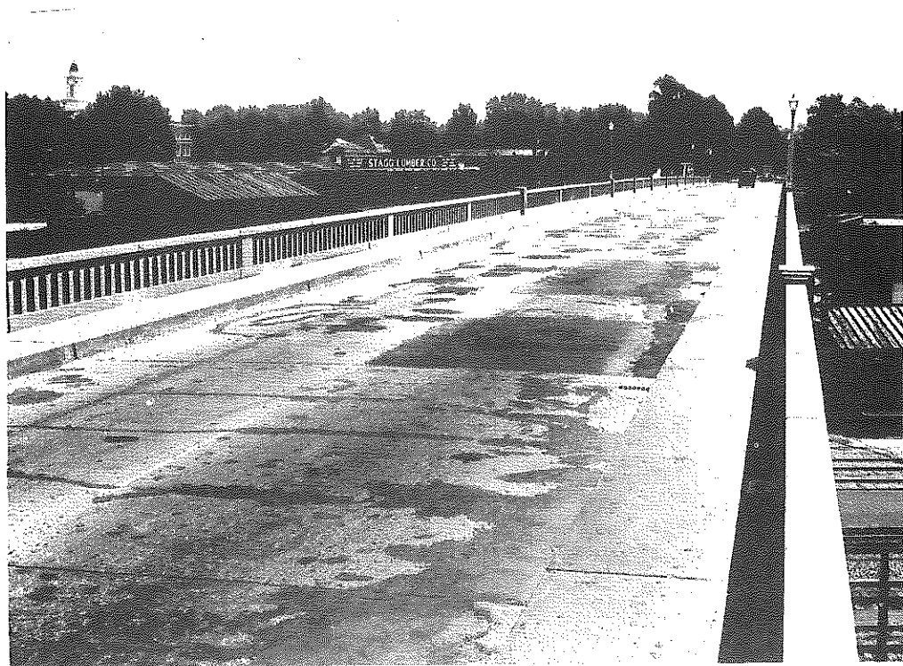
Figure 23. Bridge Deck Which Has Been Partially Restored by Patching with Tar-Modified Epoxy Resin.
