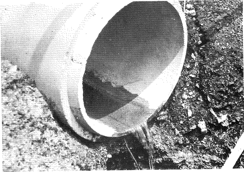
Figure 11. Concrete Pipe After 28 Days in Test at Mortons Gap.
