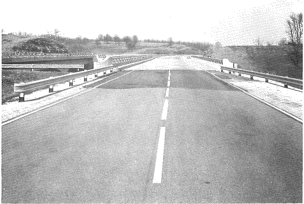
Figure 32. Patching Work often Required at Bridge Approaches to Maintain Desirable Riding Qualities and Safety.
