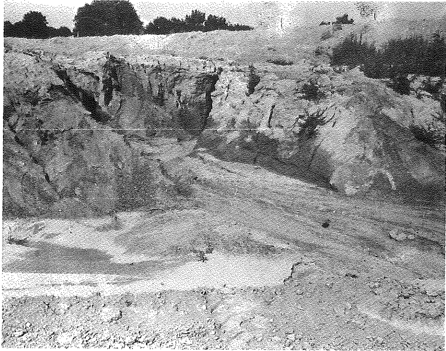
Figure 36. Photograph Showing Area of Wind-Blown Silt where Erosion Control and Stability Problems were Encountered during Construction.
