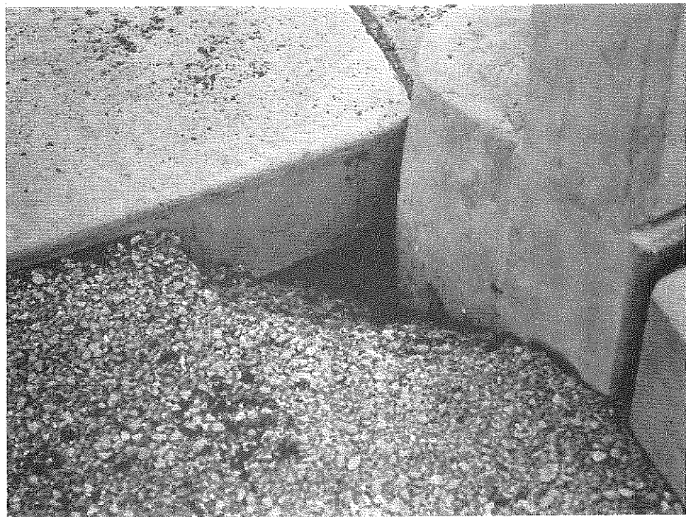
Figure 31. Development of a Void at Bridge Abutment that often Attends Settlement of Bridge Approach Slab.
