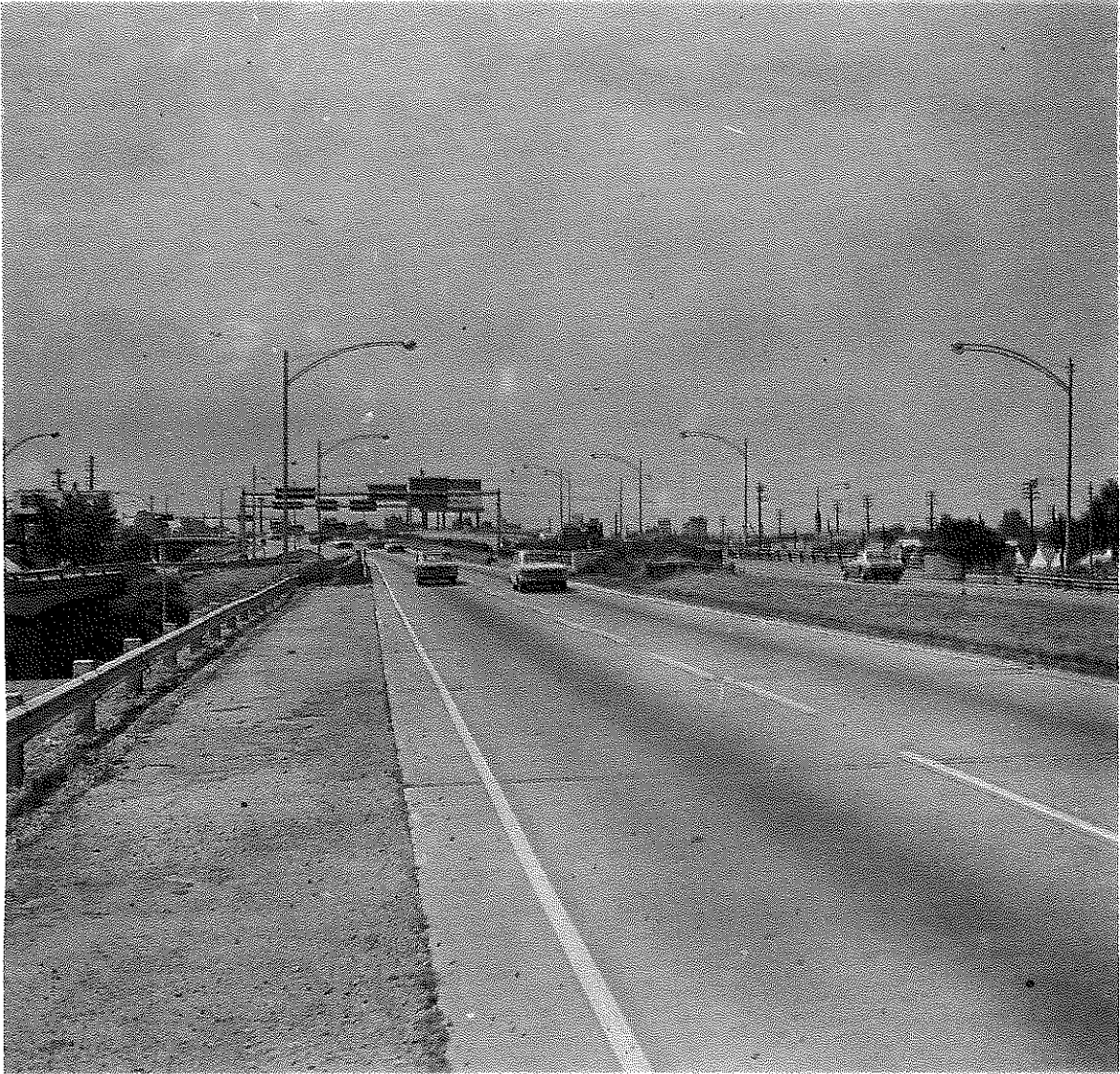
Figure 3. Portion of Test Site 8 Showing Irregular Alignment of Edge-Lines.
