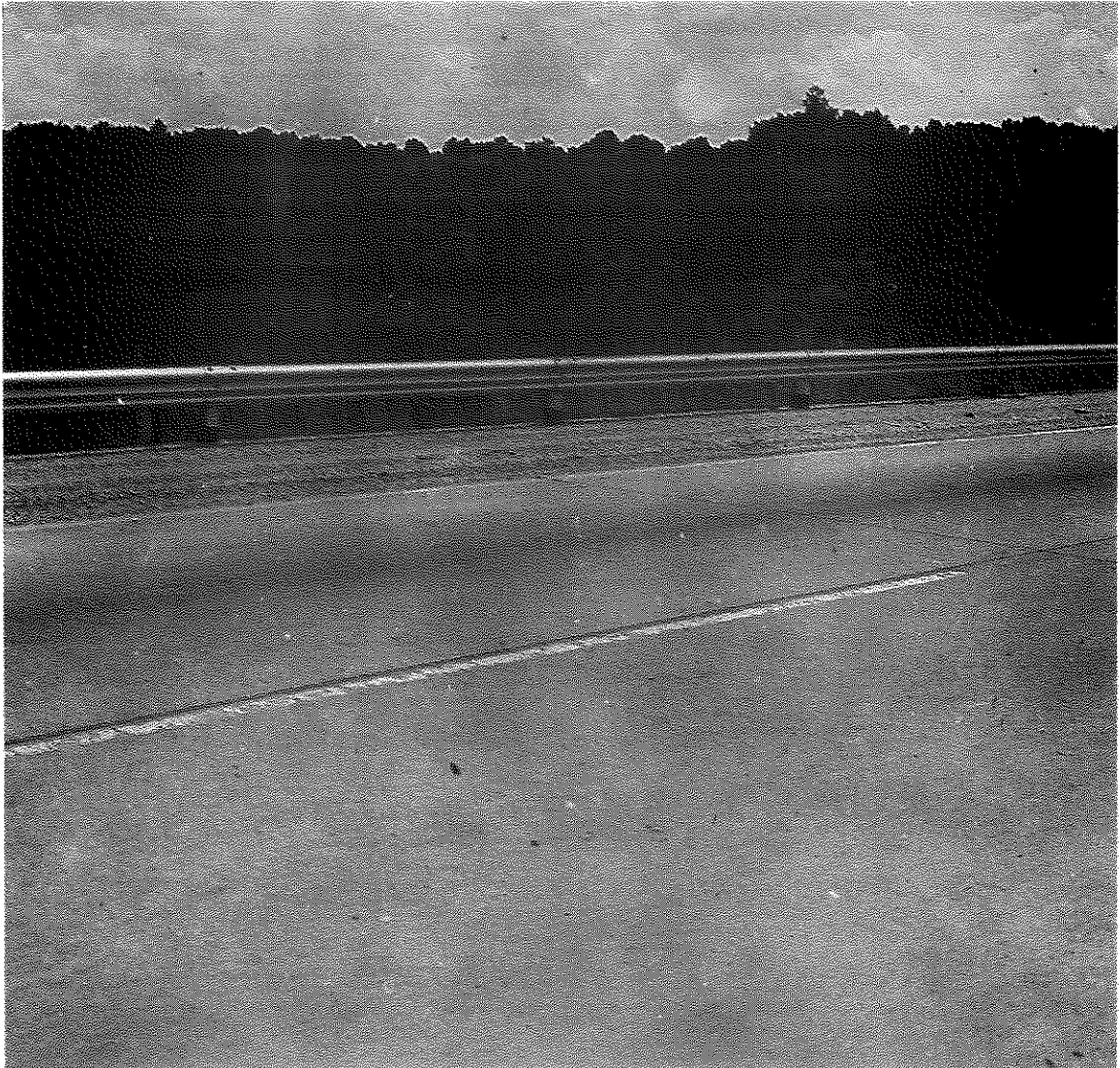
Figure 12. A Portion of the Catathern Subsection, Test Site 3, I 64, Shelby County during April, 1965. Note extreme spalling of center-line and edge-line.
