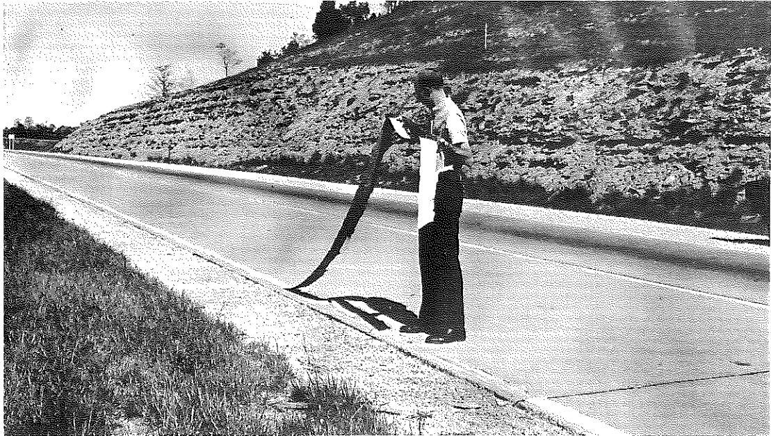
Figure 9. Photograph Showing Poor Bond of Thermoplastics in Test Site 3, I 64, Shelby County. In many areas, portions of line as long as 10 feet could easily be pulled up by hand.
