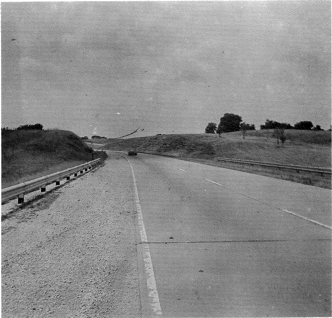
Figure 8: View of East-bound Lane of Test Site 3, I 64, Shelby County, showing a Portion of Subsection 1, Perma-Line. Photograph was taken during April, 1965 and shows spalling of the edge-line receiving drainage.
