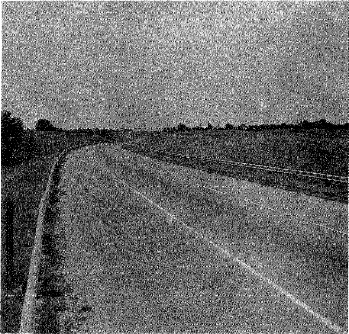
Figure 11. A Portion of the Kentucky Paint (Control) Section in Test Site 3, Eastbound Lanes I 64, Shelby County (Looking West). Since the original installation in 1962, the center-lines have been repainted three times and the edge-lines have not been repainted. Note contrasting quality of inside and outside edge-lines. Photograph was taken during April, 1965.
