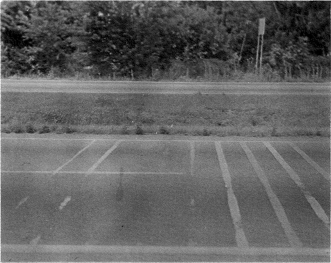
Figure 6. Transverse Lines on Bituminous Concrete Pavement in Test Site 2, I 264, Jefferson County. Lines were placed in November, 1962, and photograph was taken during July 1966. The Kentucky paint lines have not been repainted. Some minor edge spalling can be seen in lines 9 and 10. First 6 lines are Kentucky white and yellow paint--1, 2, and 3 applications, respectively; lines 7 and 8 are Perma-Line; and lines 9 and 10 are Catatherm.
