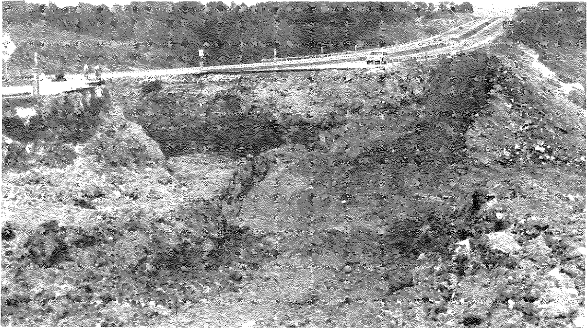
Figure 10-4. Slide Area with Unstable Material Removed.
