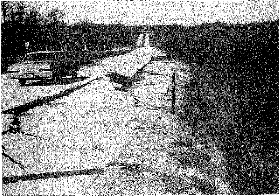
Figure 3-5. Slide at Mile Post 83, Western Kentucky Parkway, in May, 1966.
