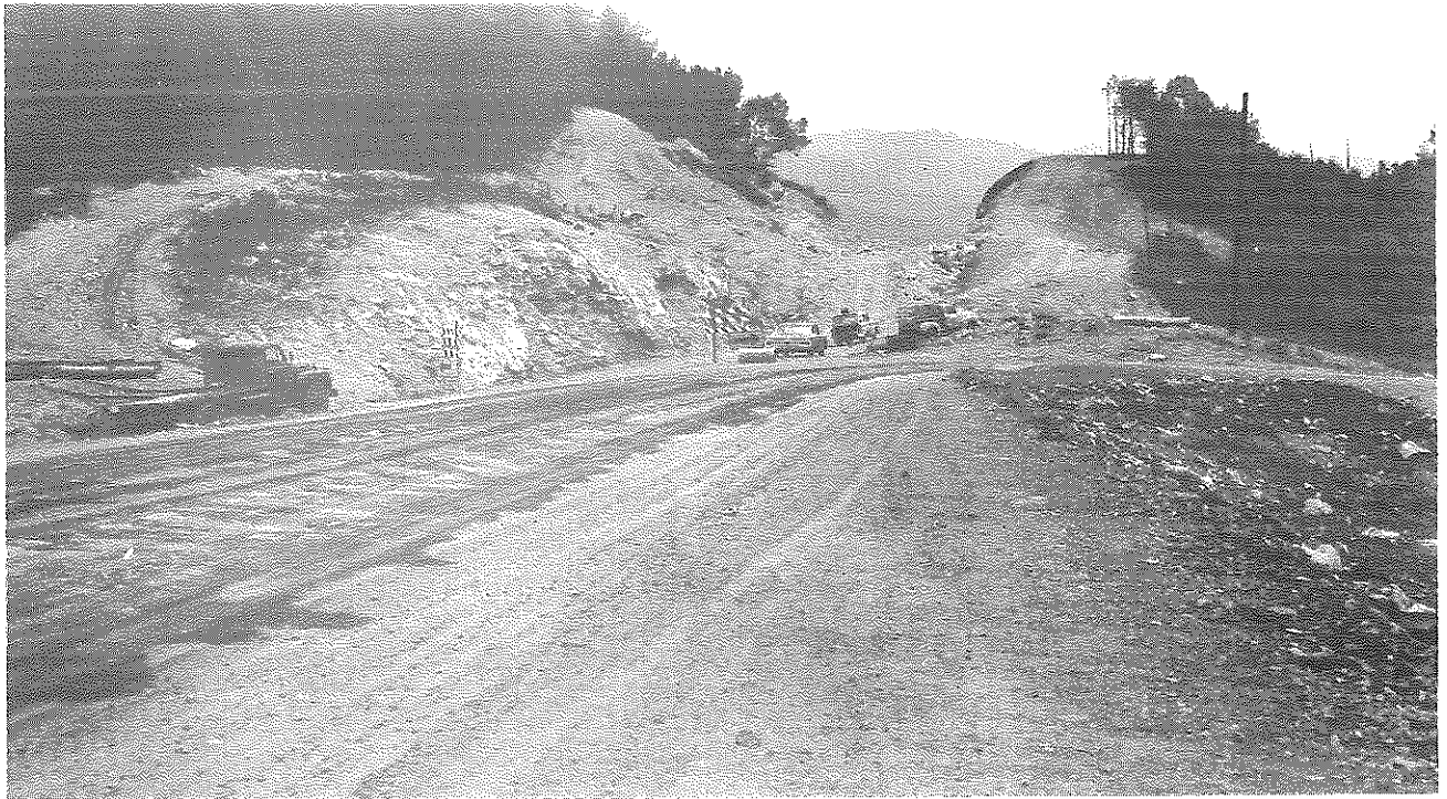
Figure 6-1. View of the Slide Area From the Southwest.
