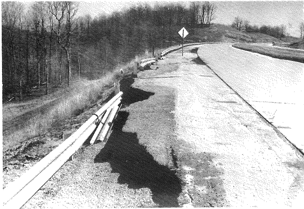
Figure 3-2. Slide at Mile Post 83, Western Kentucky Parkway, in February, 1966.
