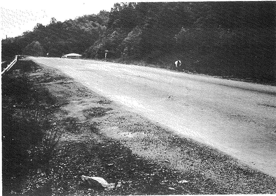
Figure 4-2. View of Slide Area Showing Displacement of Guard Rail.
