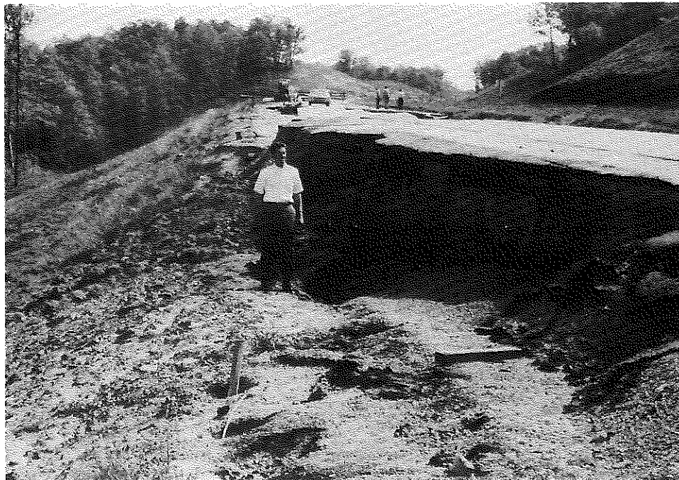
Figure 3-4. Slide at Mile Post 83, Western Kentucky Parkway, in May, 1966.
