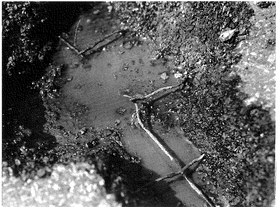
Figure 2. Close-up View Showing Deteriorated Condition of Wire Mesh.
