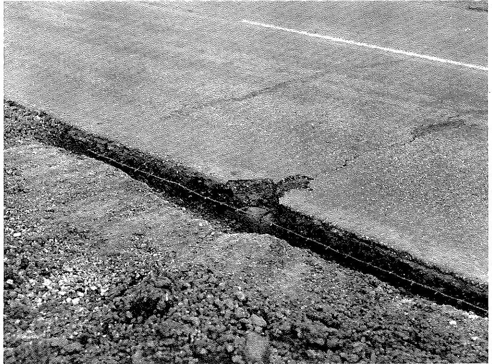
Figure 3. View Showing Reflection Crack over Joint in Rigid Slab and Associated Crack at Edge of Wire Mesh Reinforcement.
