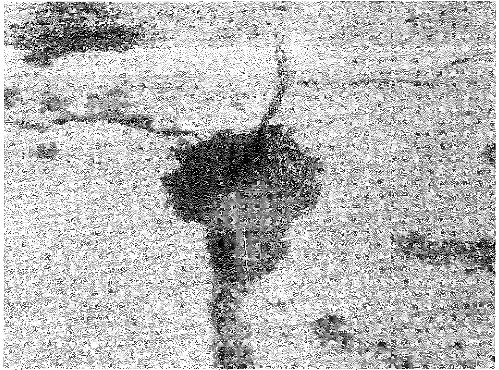
Figure 1. Exploration Hole to Study Condition of Wire Mesh.
