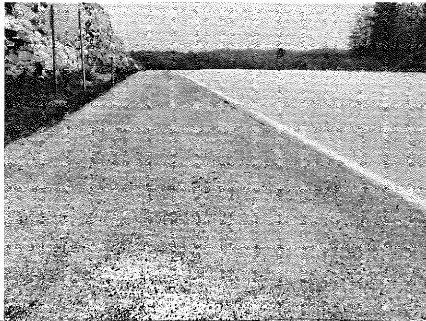
Figure 6. Cement-Treated Section Near Mile Post 44.49, May 1, 1968. This was one of the most severely distressed areas of shoulder.
