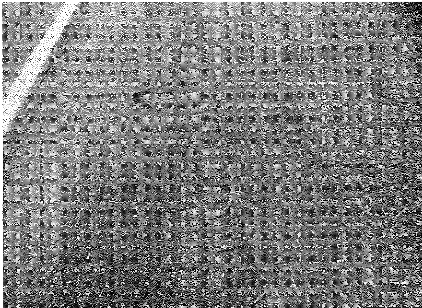
Figure 10. A Rutted and Cracked Area in the Cationic Emulsion Treatment, May 1968.
