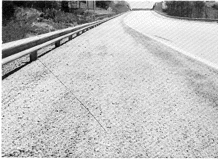
Figure 5. Typical Appearance of Cement-Treated Section near Mile Post 44.18, May 1, 1968. Note the dark strip next to the pavement where the seal was shaved by snow removal equipment.
