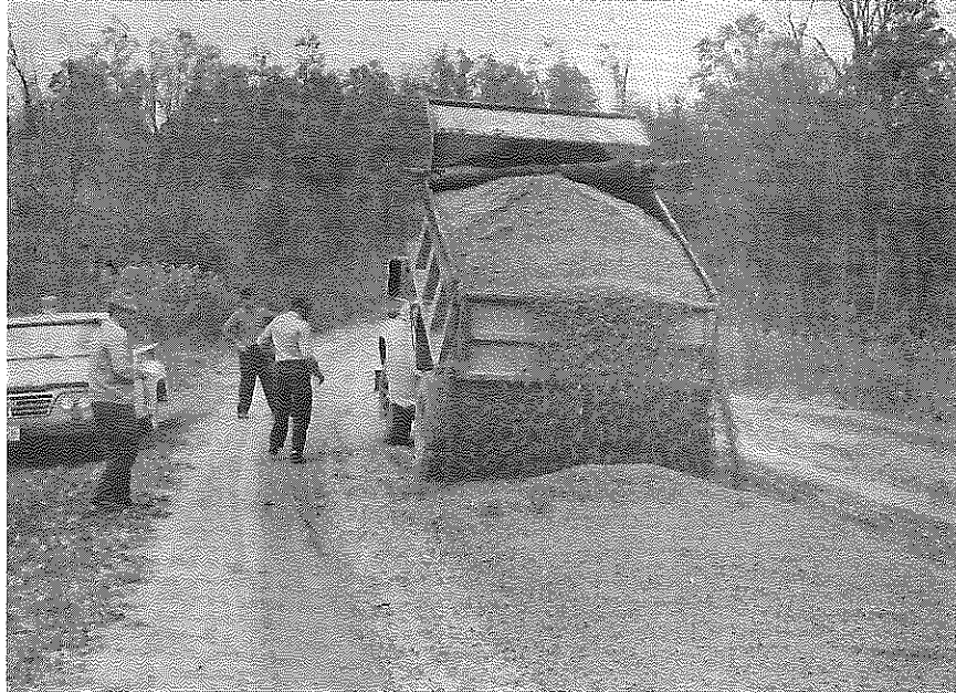
Fig. 7. The Aggregate was Spread on the Roadway by Tailgating the Aggregate Over the Proper Distance.
