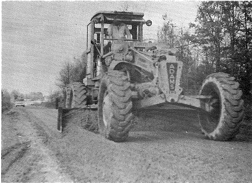
Fig. 8. The Material was Manipulated Across the Full 16-foot Width with a Patrol Grader. A sharply defined edge was gained by use of stringlines and a cut-off on the grader blade.
