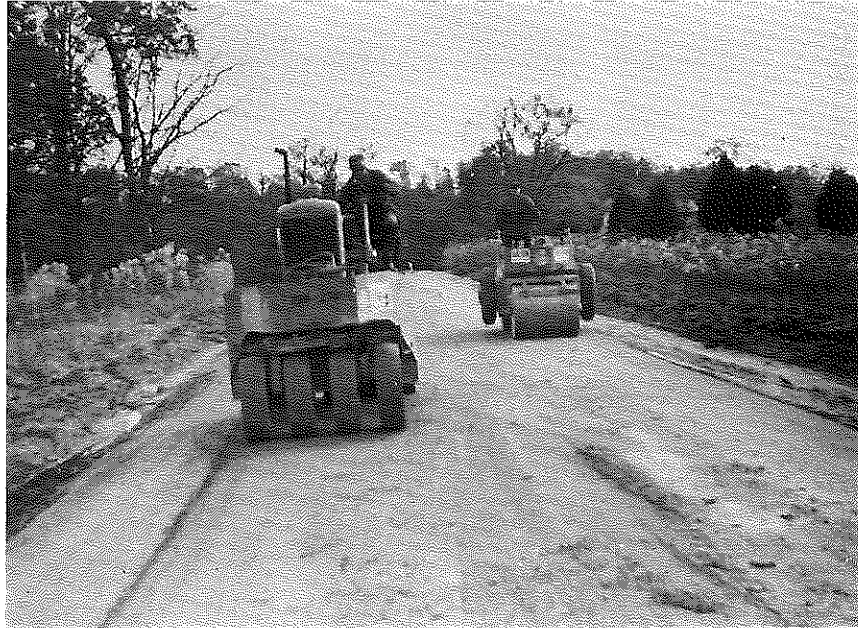
Fig. 9. Pneumatic-Tired and Steel-Wheeled Tandem Rollers Compacting DGA Base. The rollers were kept moving during the placing operations and good density was obtained.
