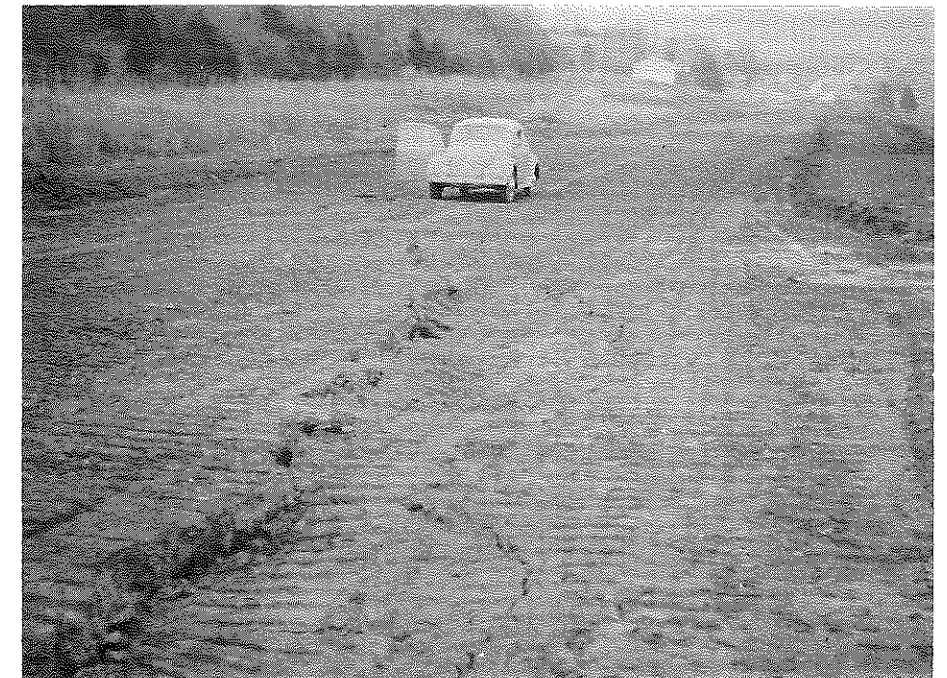
Figure 8. Distress in Embankment on KY 52, Estill County (December 1967).
