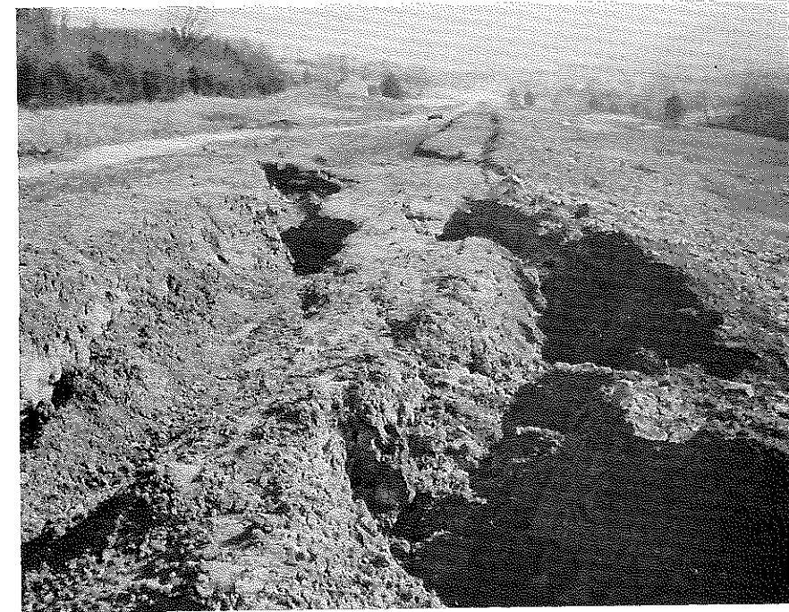
Figure 10. Distress in Embankment on KY 52, Estill County (February 1968).
