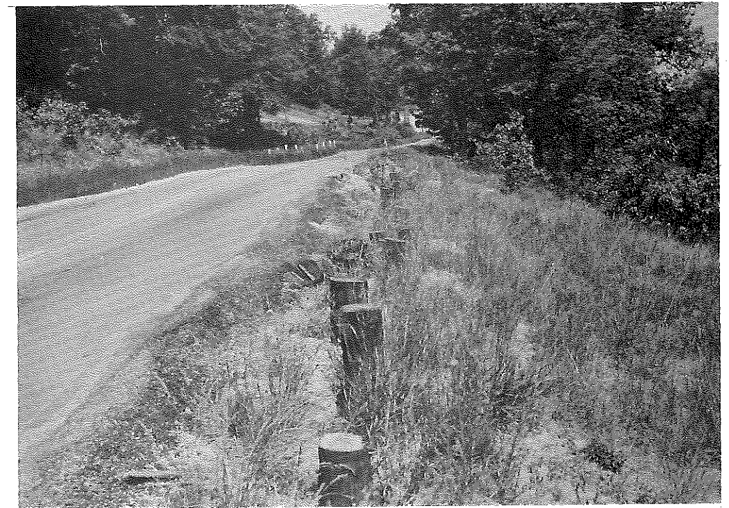
Figure 18. Photograph 2 (See Figure 15) of Slide Area, KY 89, Clark County.
