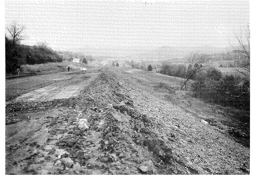
Figure 7. View of Landslide Site on KY 52, Estill County (December 1967).
