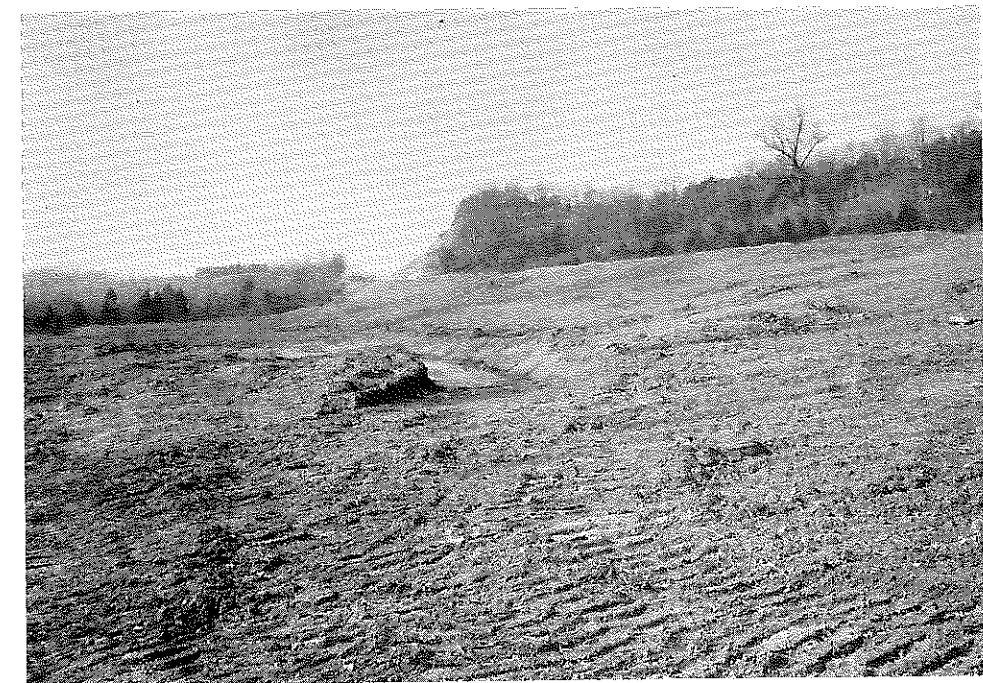
Figure 11. Distress in Embankment on KY 52, Estill County (February 1968).
