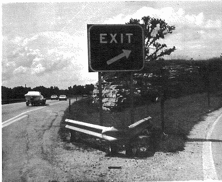
FIGURE 39. Location 10; Fayette County, I 75 - US 25 and US 421 Interchange, Gore at Northbound Exit from I 75 to US 25 and US 421
