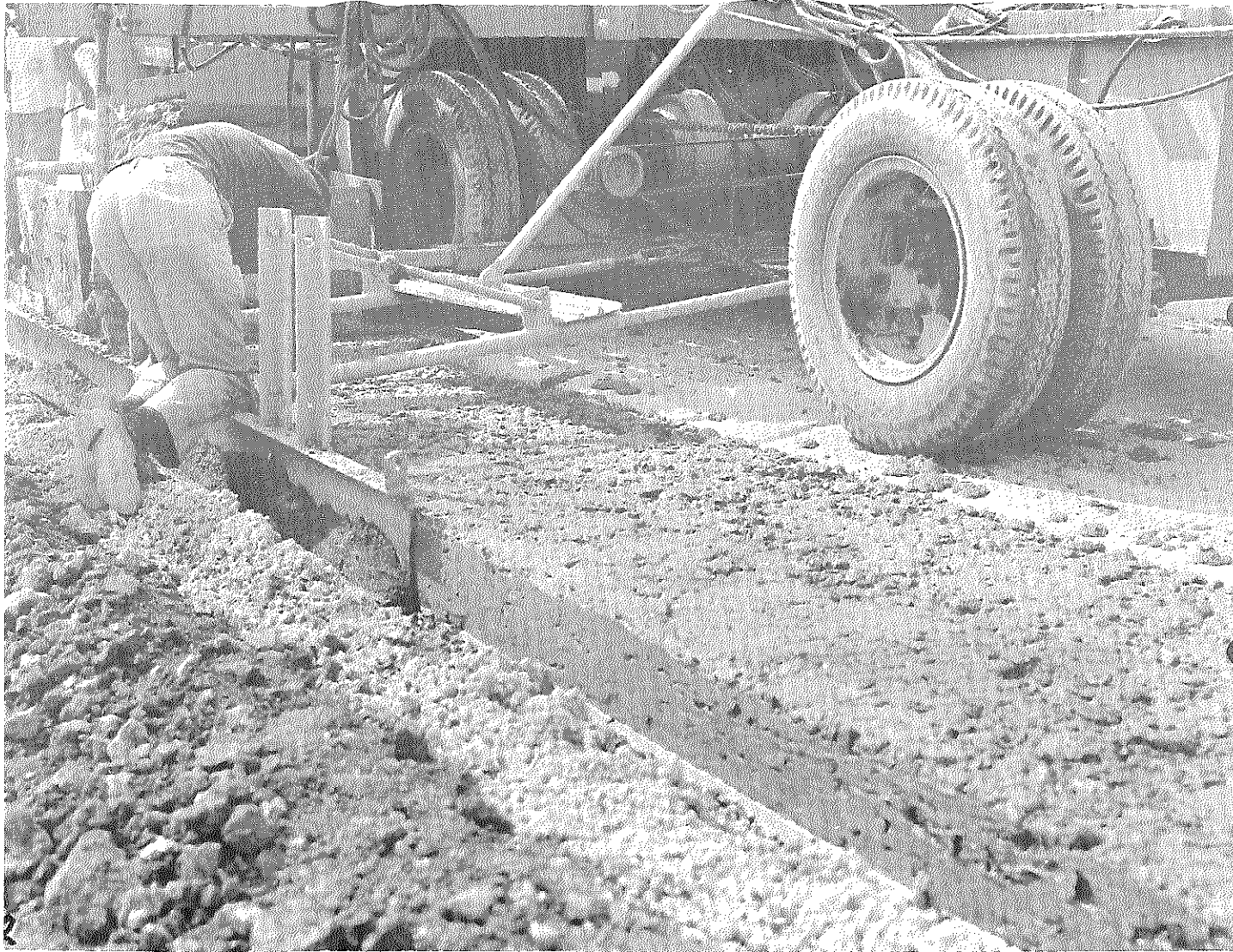
Figure 2. Close-up View of Slip-Form Paver on Lexington-Versailles Road. Note Vertical Edge of Low-Slump Concrete.
