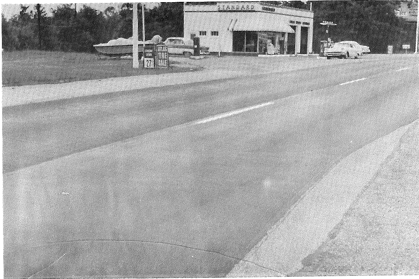
Figure 13. US 60, Shelbyville to Middletown, September 1963. A view of a section of the four-lane pavement shortly after sealing.
