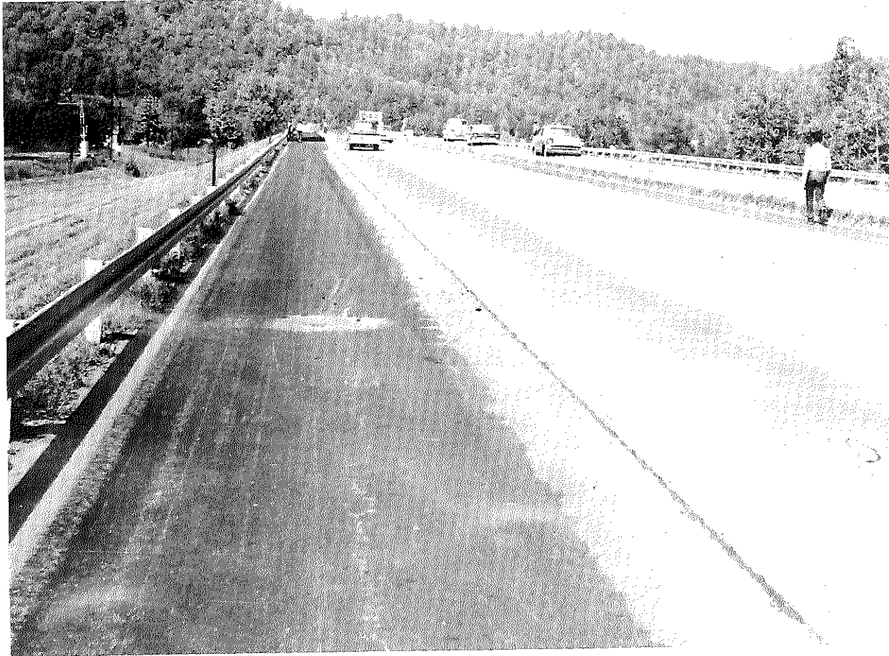
Figure 16. Kentucky Turnpike, Louisville to Elizabethtown, September 1963. A typical view of an outer shoulder just prior to sealing.
