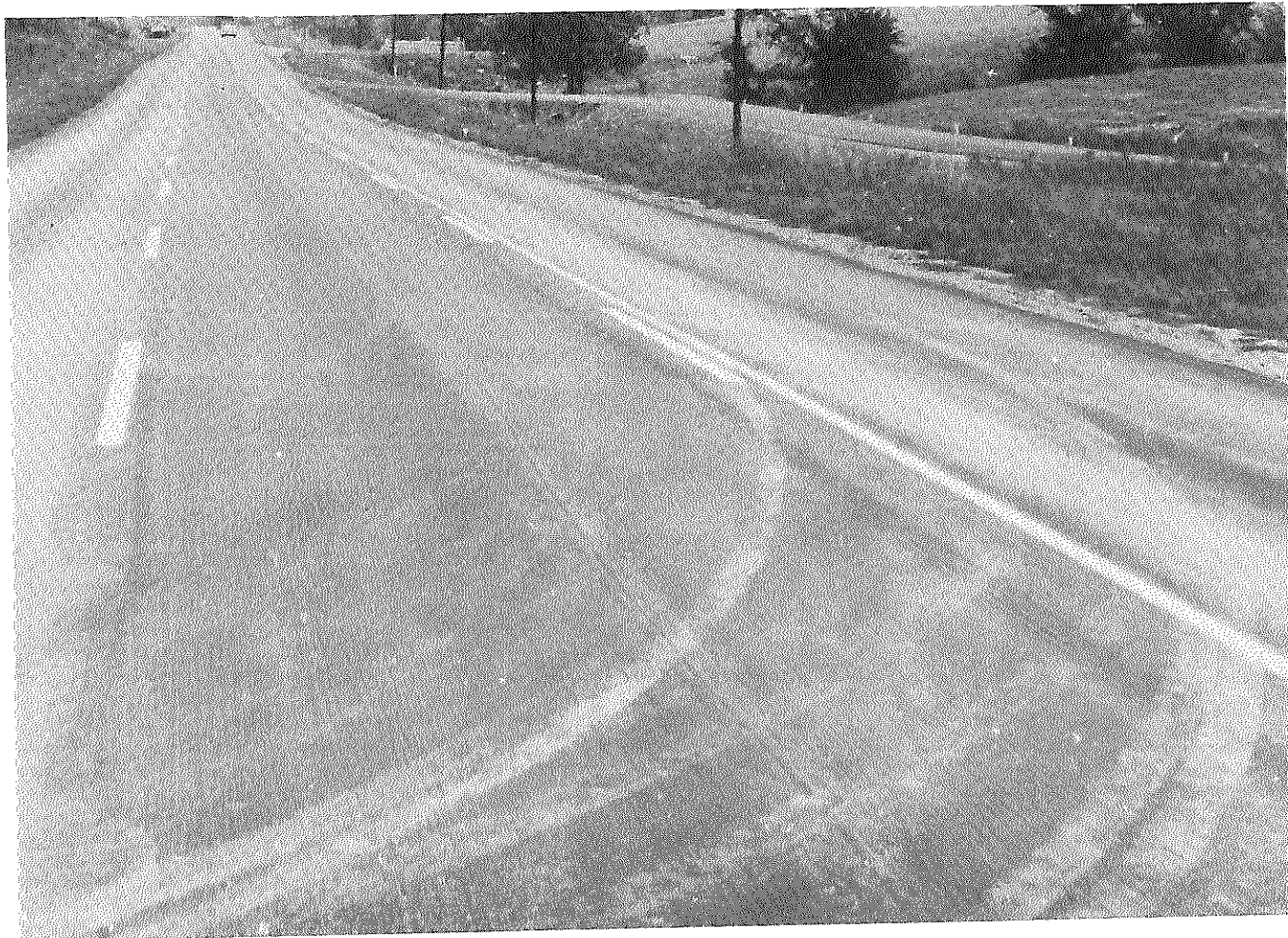
Figure 27. US 60, Shelbyville to Frankfort, July 1965. Note the glazed appearance in the wheel tracks of the outer lanes.
