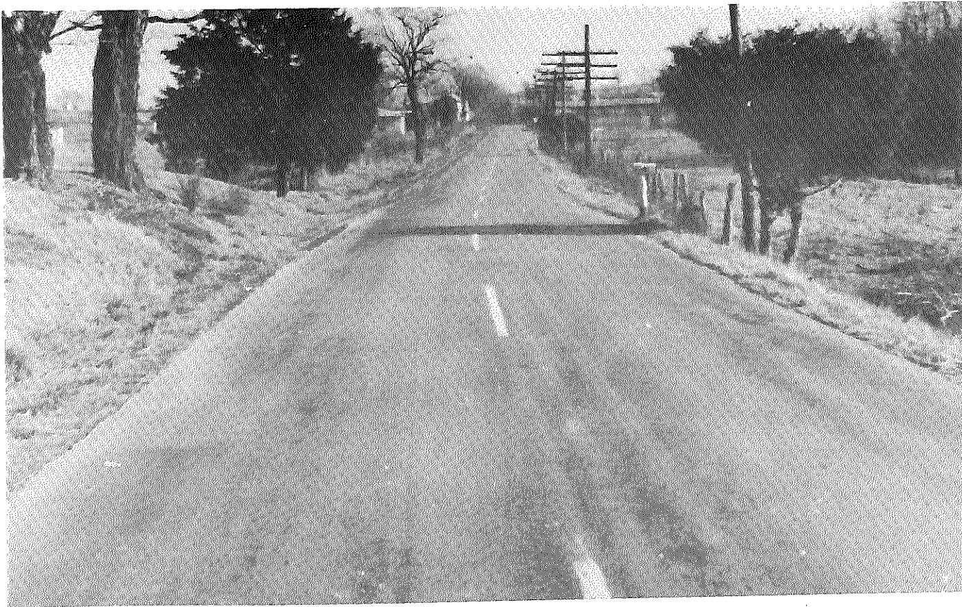
Figure 23. . US 68, December 1966. Typical appearance of the roadway two and one-half years after sealing.
