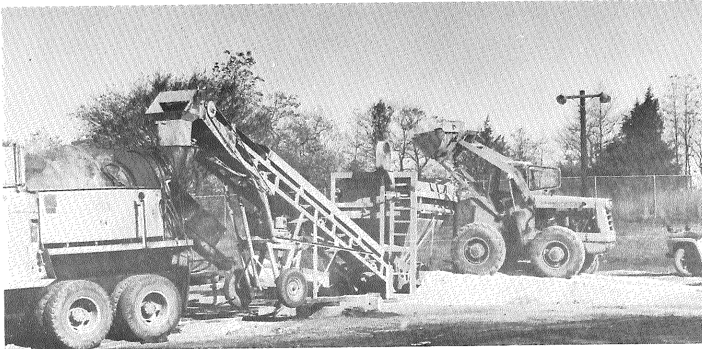
Figure 1. View of Ross Porta-Plant used to proportion slurry seal aggregates and water.
