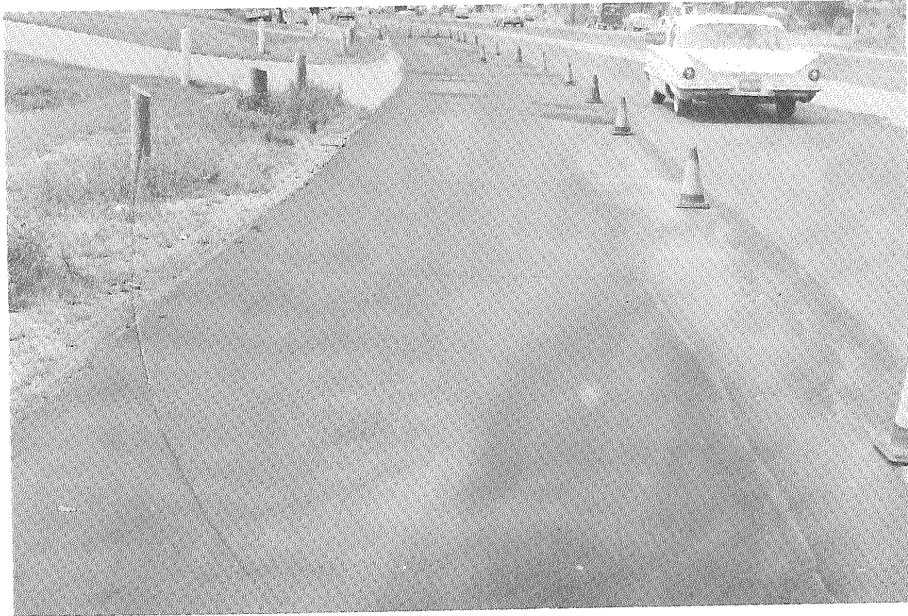
7 Figure 5. An example of traffic cones placed to keep traffic off a fresh application. Note the tire marks in the seal from side entrance traffic and the wetter appearance of the seal in areas that were laid thicker.
