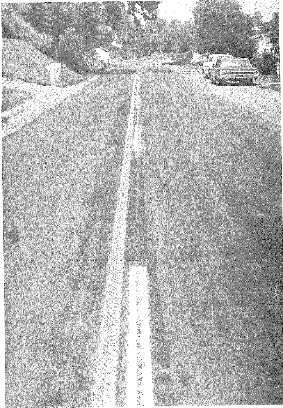
Figure 25. KY 5, Boyd County, August 1965. A view of the roadway shortly after sealing. Difficulty was experienced with a premature break of the emulsion.
