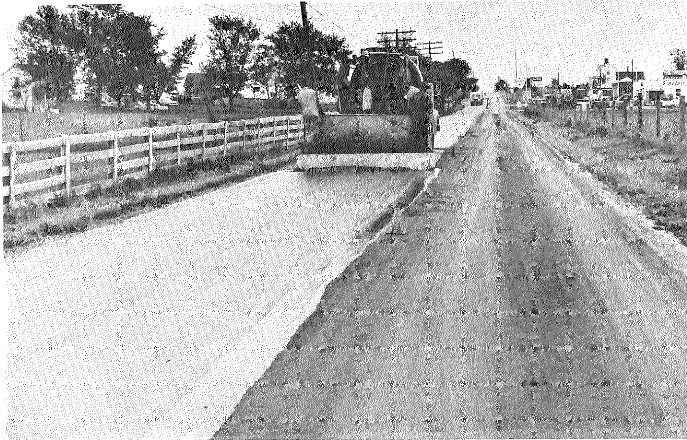
Figure 28. US 27 at Nicholasville, May 1966. An excess of emulsion in this mixture was a result of a leaking valve in the asphalt proportioning equipment. The seal was cured two hours before allowing traffic onto the surface.
