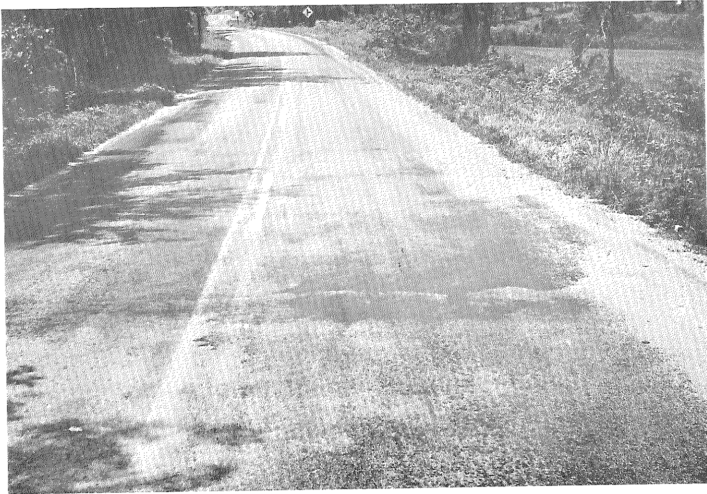
Figure 20. US 68 at the Boyle-Mercer County line, June 1964. Typical appearance of the roadway prior to sealing.
