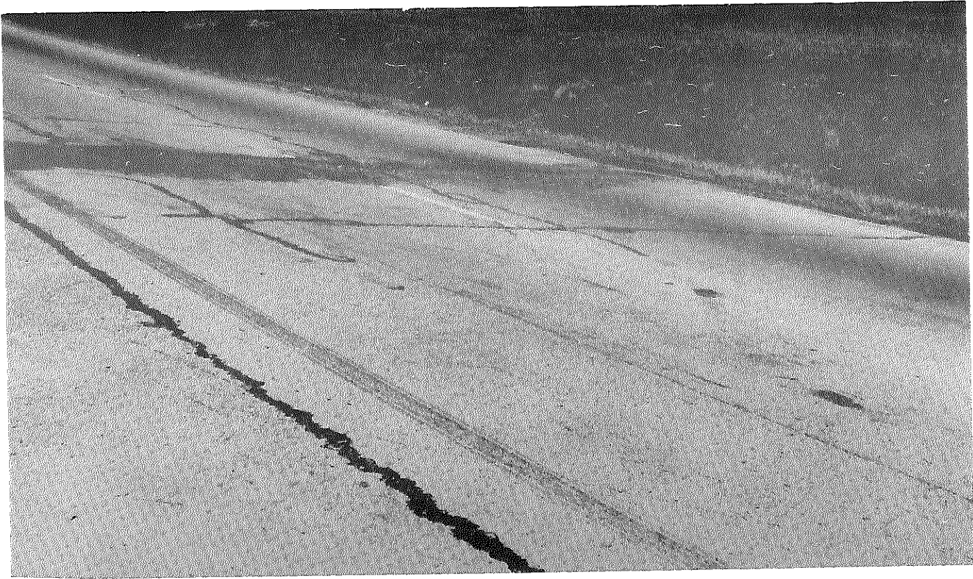
Figure 11. US 60, Shelbyville to Middletown, August 1963. A typical view of the appearance of the surface before sealing. Note the area where excess bituminous material was shaved off a rough transverse joint.
