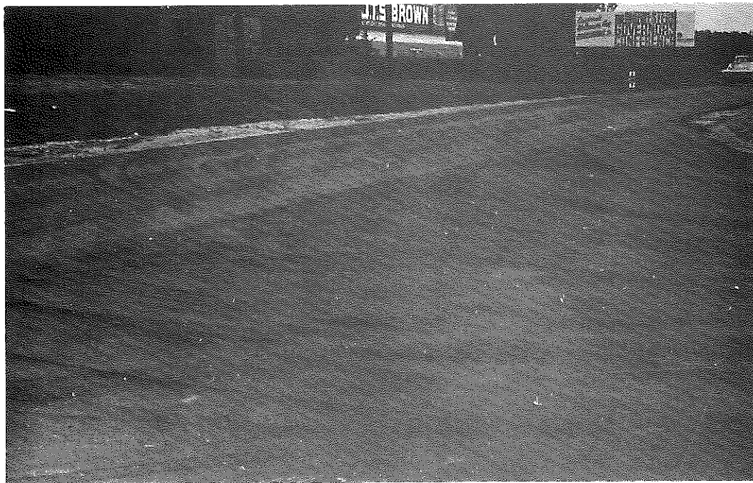
Figure 2. Greater Cincinnati Airport Entrance. Note the raveled surface in the foreground. A midrange production temperature, fly ash mineral filler, and absence of silicone in the asphalt cement combined to produce a mixture susceptible to damage by traffic.
