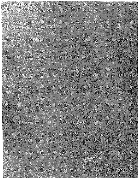
Figure 18. 12th Street in Covington. Mat tears caused by dragging paver screed.
