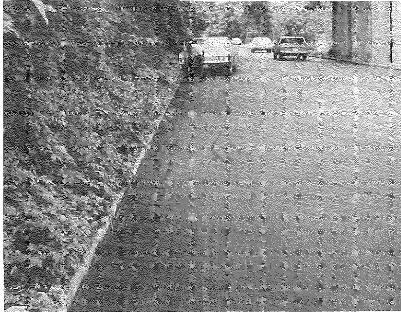
Figure 20. Lafayette Drive in Frankfort. Area next to curb appears to have been hand compacted.
