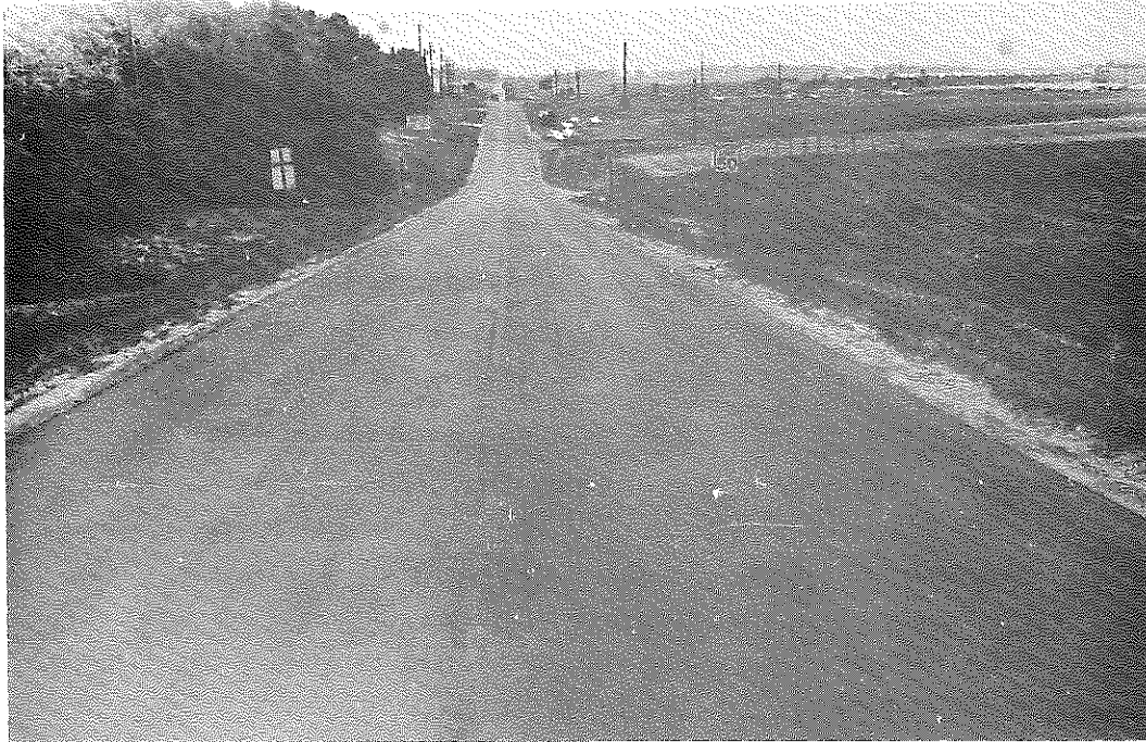
Figure 1. Greater Cincinnati Airport Road. The flushed appearance in the wheel tracks is attributed to the fly ash mineral filler.
