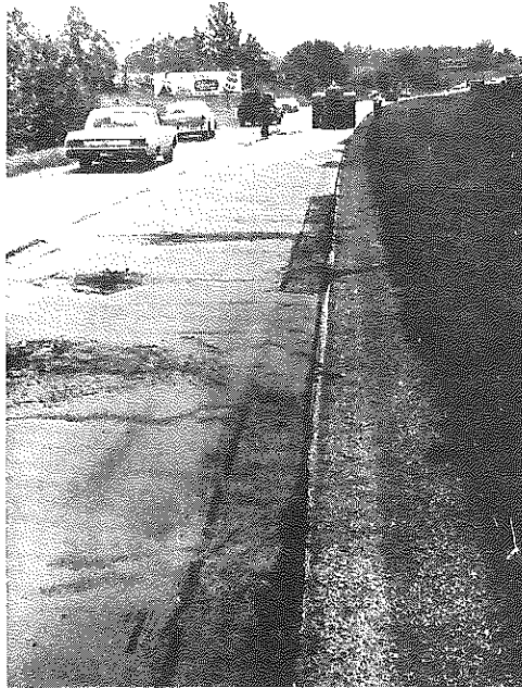
Figure 9. US 41, Hopkins County. The lack of silicone and high moisture content in the aggregate combined to cause bubbles, mat tearing, and segregation in the sand asphalt. Considerable handwork repairs were required.
