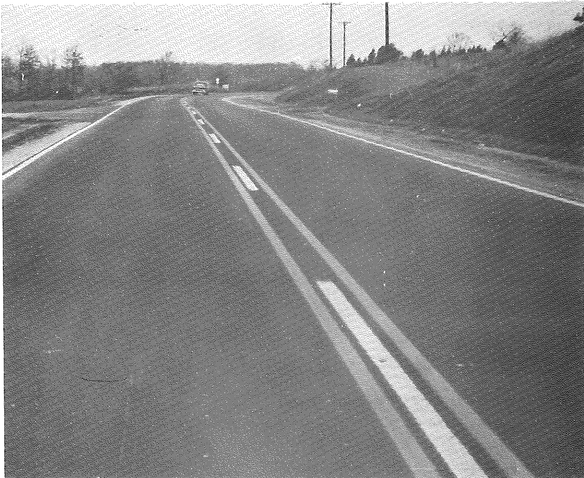
Figure 23. US 27, Somerset. Note scaling in the wheel track of southbound (left) lane.
