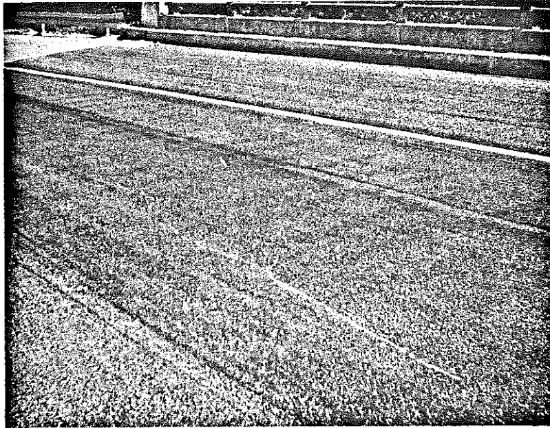
Figure 7. Soft Area in Northbound, Outside Travel Lane on the Clear Creek Bridge (Only Soft Area Noticed).
