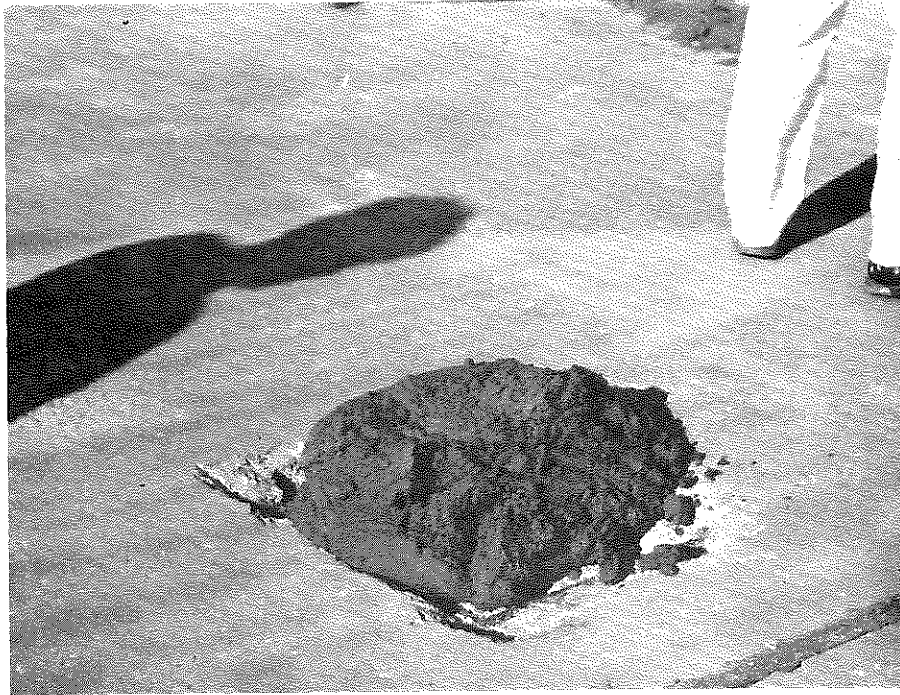
Glazon is Used to Patch Areas Where Deteriorated Concrete Has Been Removed.
