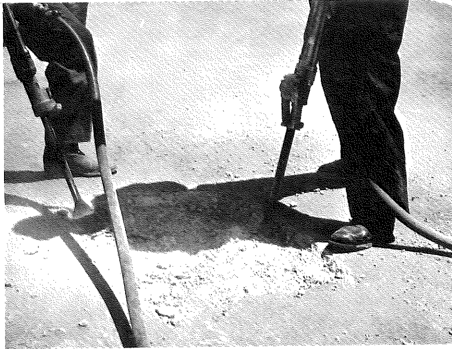
Deteriorated Concrete is Removed by Use of 35-Pound Pavement Breakers in Preparation for Glazon.
