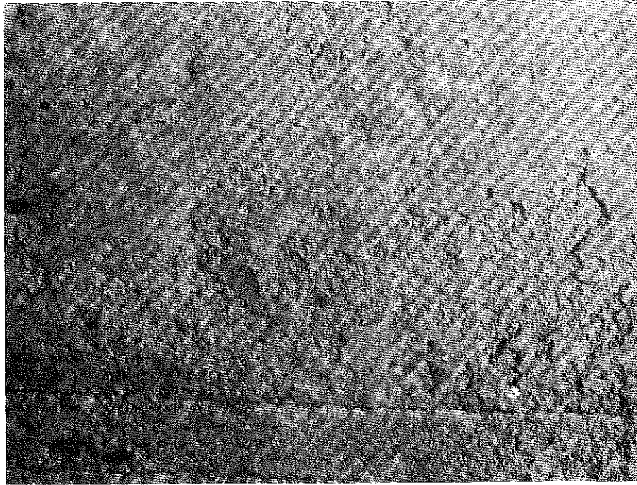
Figure 16. Deterioration on the Clay City Deck, December 29, 1971
