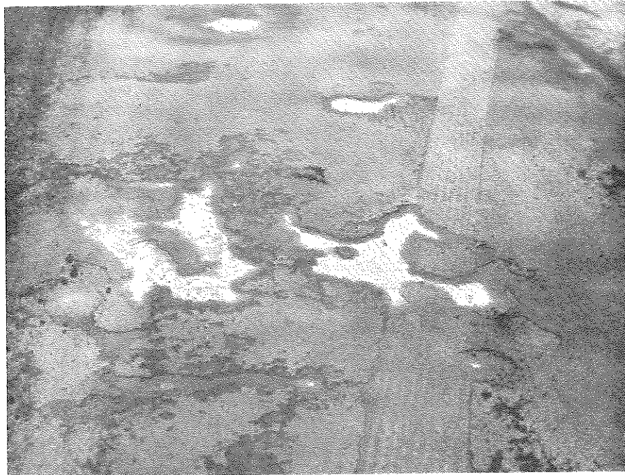
Figure 13. Peeling and Deterioration of Overlay on the Shelby County Bridge
