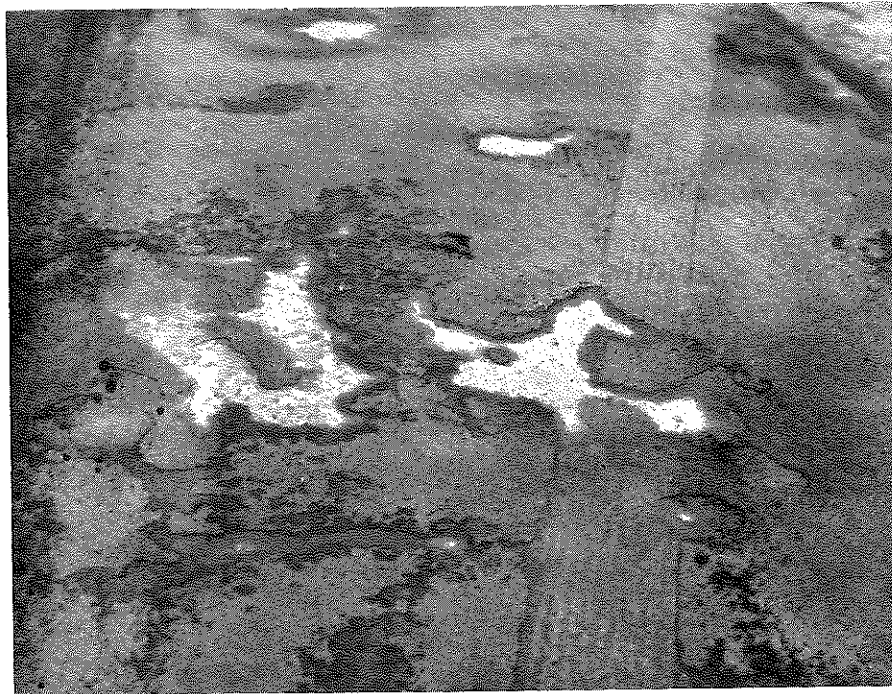
Finished Product on Bridge Carrying KY 395 over Westbound I-64 Three Days after Completion. Note Failure.
