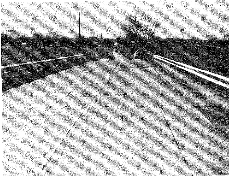
Figure 20. General Appearance of the Clay City Bridge Deck, December 29, 1971
