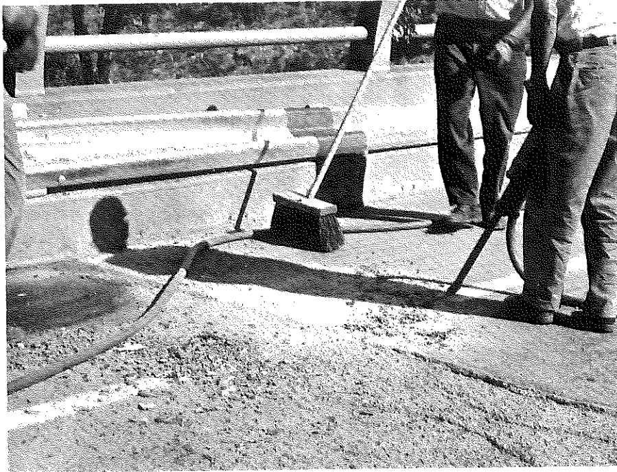
All Blacktop, Loose Sand and Other Foreign Material is Removed in Preparation for Glazon.
