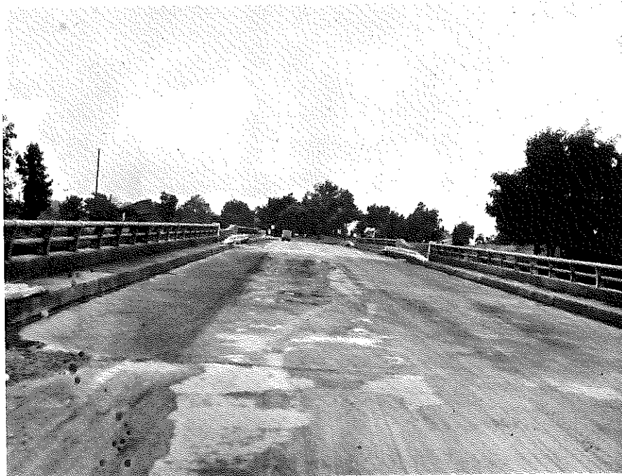
Finished Product on Bridge Carrying KY 395 over Westbound I-64 Three Days after Completion. Note Failure.
