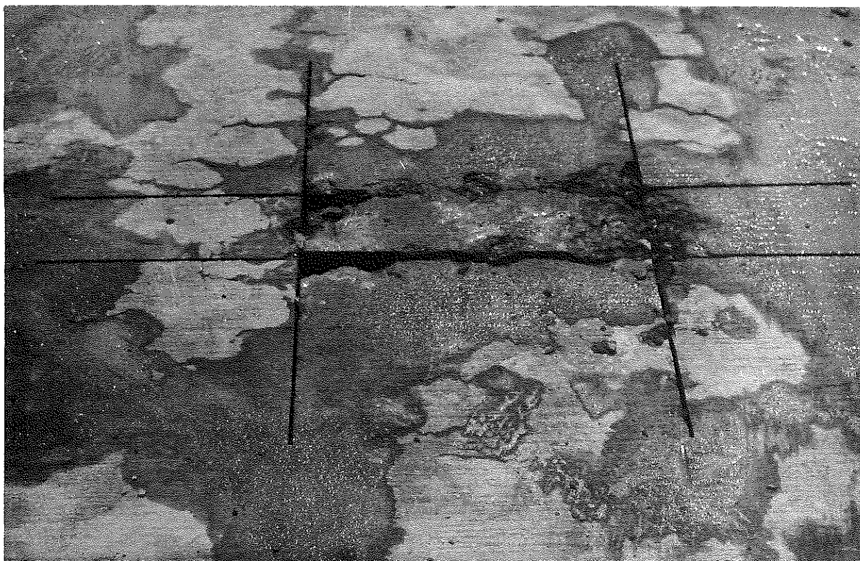
Figure 15. Gage Points Set in Pavement, Measured, then Block Sawed Free. Change in length between gage points -- due to relaxation -- was used to compute stress. Note cracking in lower photo (Station 226+00 SB).
