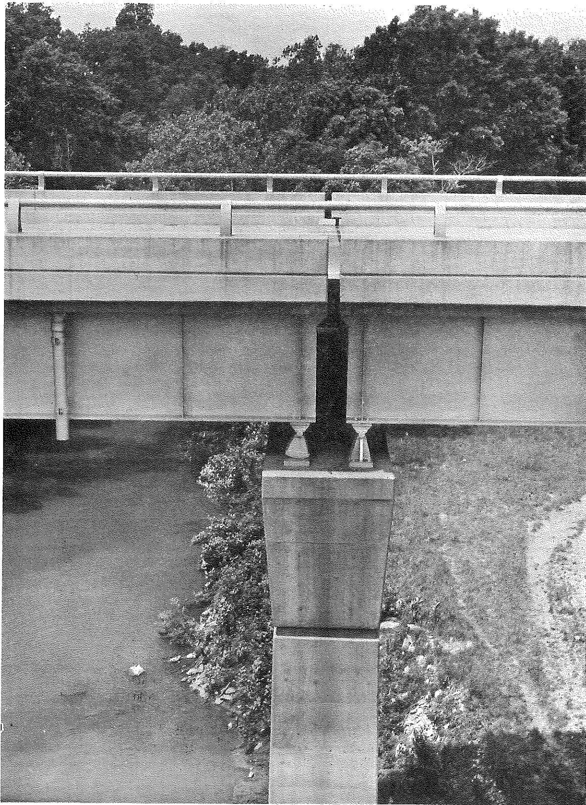
Figure 6. Bridge over Drakes Creek, I 65-1(8), Showing Northward Thrust of South Abutment and Closure at Center Pier. South abutment wall sheared, subsequently repaired; damage attributed in large part to expansion of pavement south of bridge.
