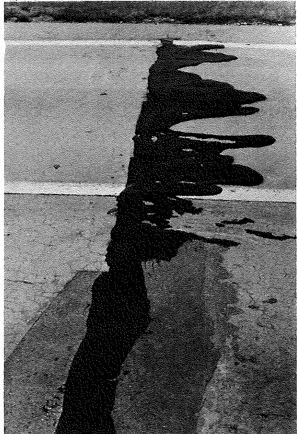
Figure 12. Rubberized Asphalt Filler Extruded from Relief Joint, near Drakes Creek, Due to Closure; March 7, 1972.
