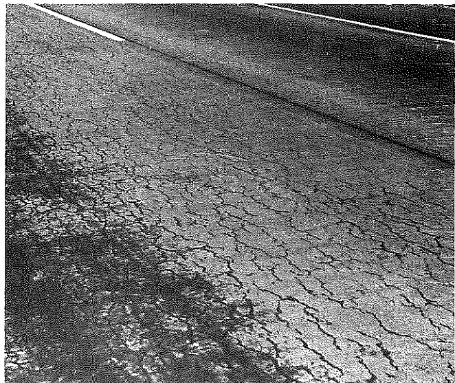
Figure 3. I 65, Crack Pattern Made Obvious by Moisture after a Rain; October 1967.
