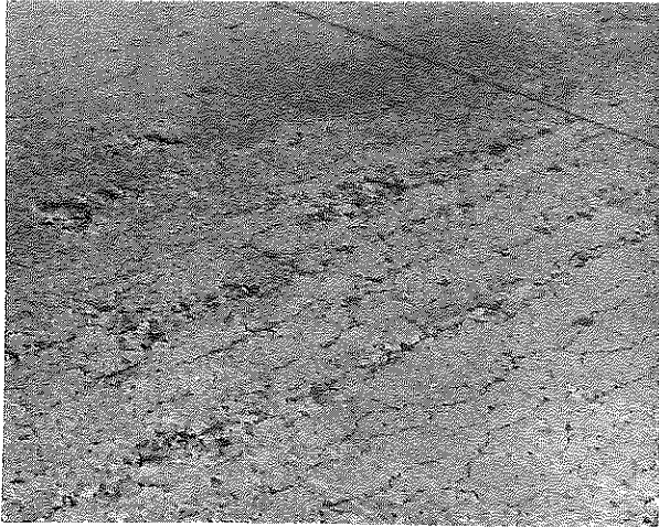
Figure 32. Advanced Cracking, I 65, MP 22, NB; March 7, 1972.
