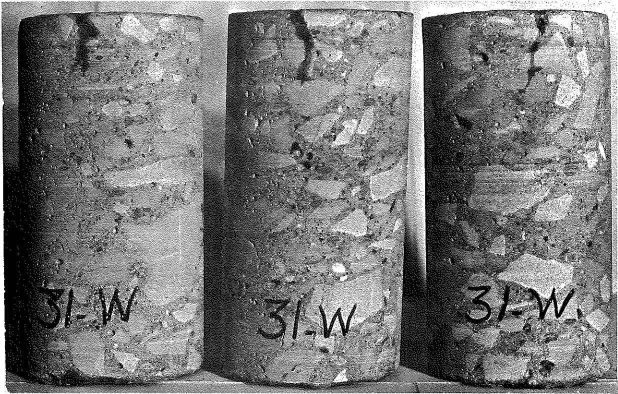
Figure 50. Cores from US 31 W North of Tennessee Line. Surface cracks are delineated by wetting. The aggregate is presumed to be from the Ste. Genevieve formations north of Franklin. Pavement was cured with a lacquer-type membrane.
