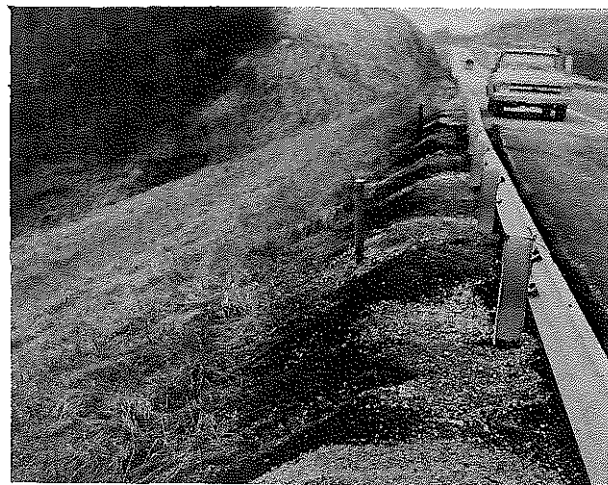
Figure 4. View of Patched Pavement.
