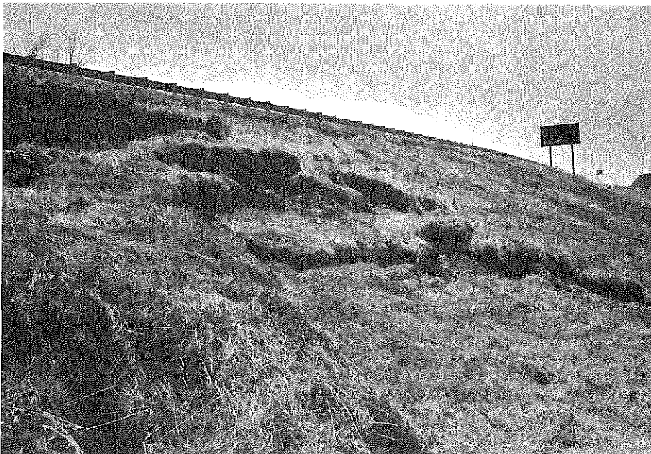
Figure 2. View of Surface Breaks Located at the Western Flank of the Embankment Failure.
