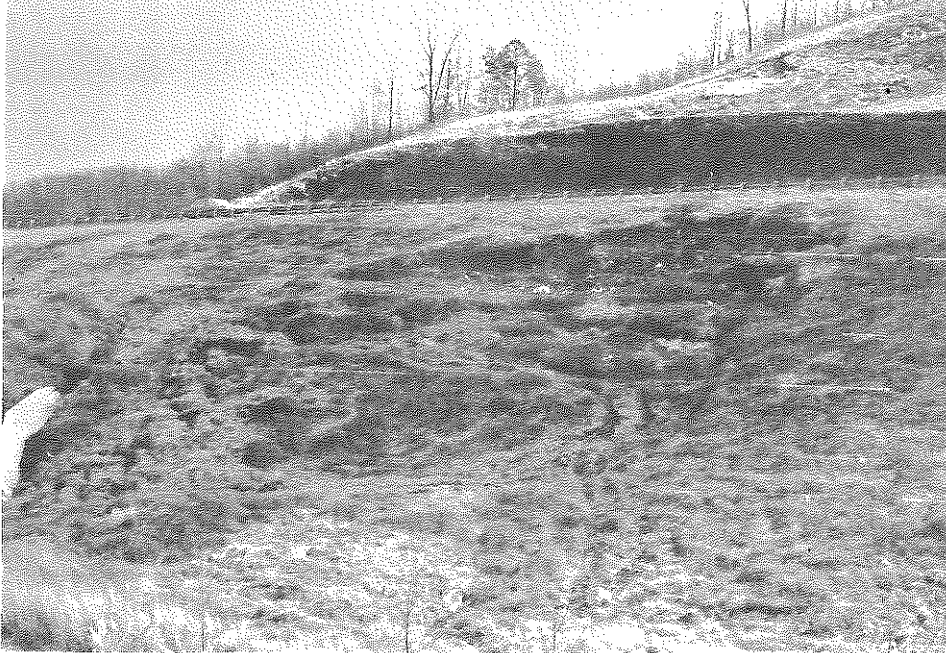
Figure 1. General View of the I-64 Embankment Failure Located Near Milepost 153, Station 3483+00.
