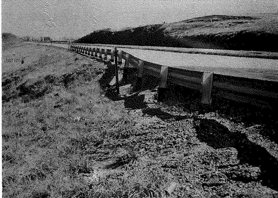
Figure 20. View of Surface Break of Westbound Lanes of Western Kentucky Parkway at Station 6922 + 50.
