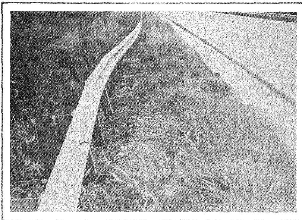
Figure 41. View of Surface Break at Inside Shoulder of Eastbound Lanes on I 64 at Station 1865 + 50.
