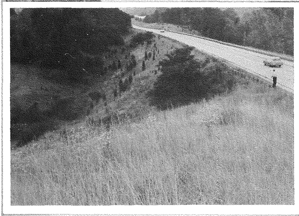
Figure 43. General View of Slide Area, Looking East, on I 64 Near Milepost 44.
