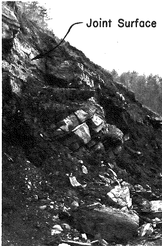
Figure 3. Failure along a Stress Relief Joint.
