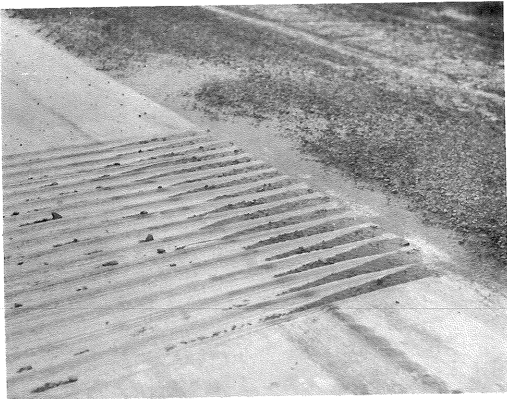
Figure A-12. Drainage Problem at Rumble Strip.
