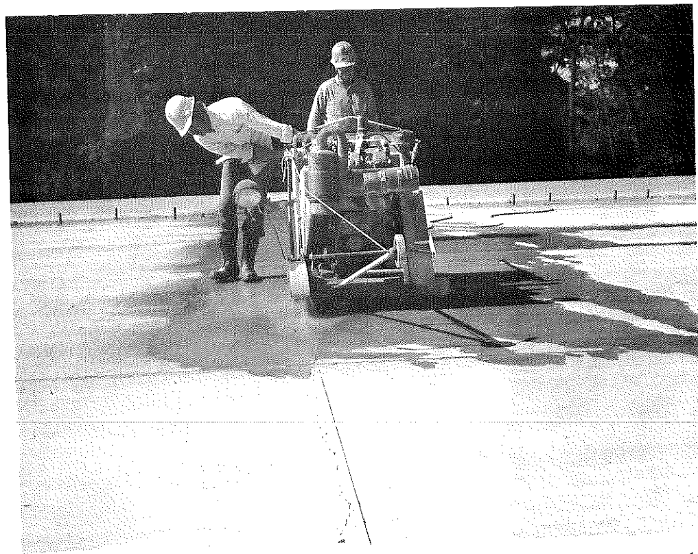
Figure A-10. Widening Joints; Note Crack in Shoulder.
