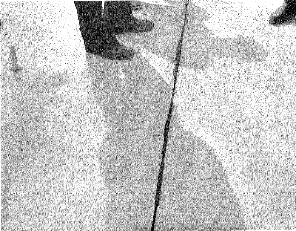
Figure A-17. Problem Area with Neoprene Seals.
