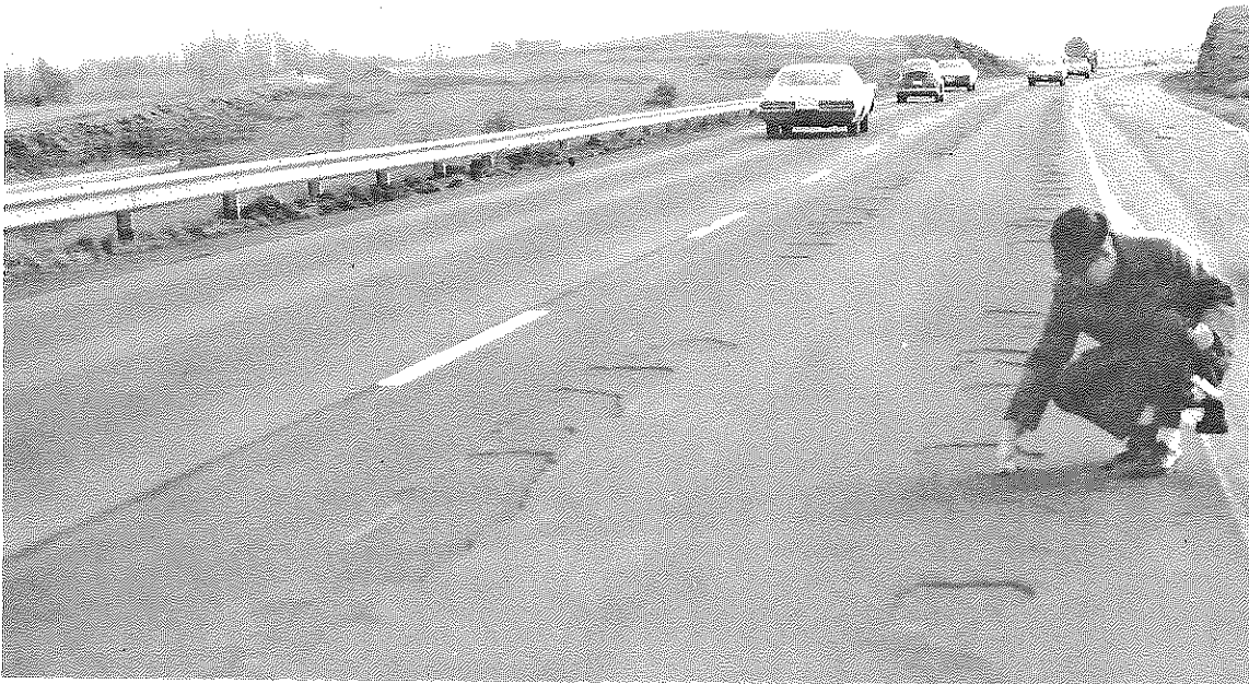
Fig. 1: Early Scaling of Sand-asphalt having Low Stability and Insufficient Asphalt.
