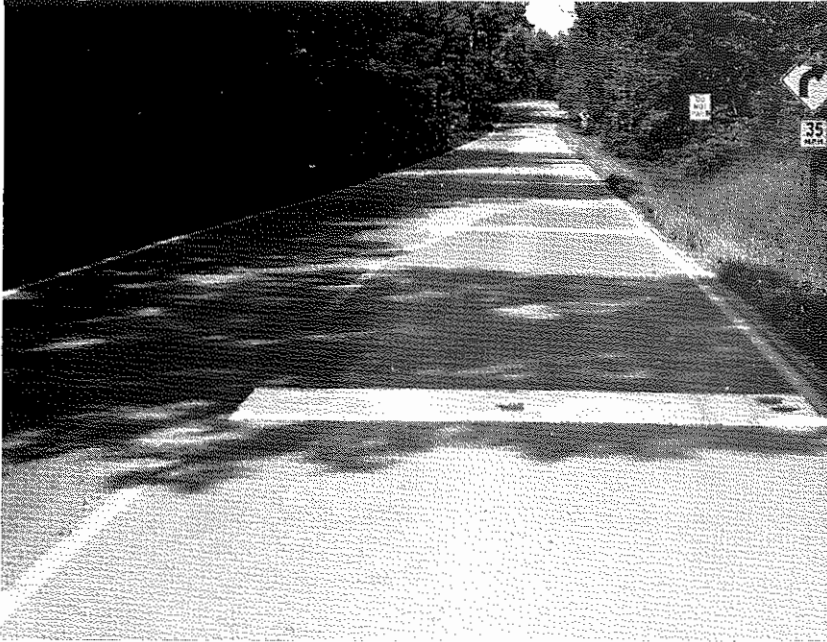
Figure 12. Test Location 1 Year after Installation of Stripes.
