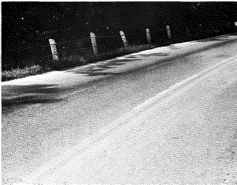
Figure 6. Guardposts Connected with Cable at the Curve.
