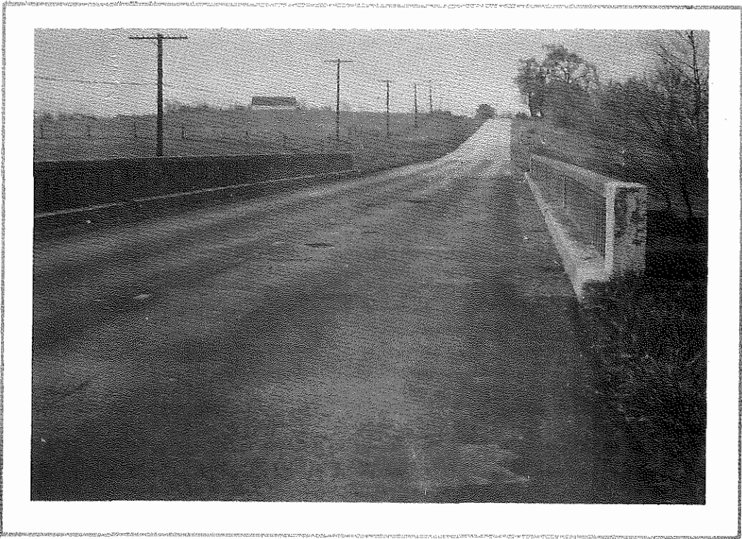
Figure 4. View of the Deck Showing Numerous Pot-Holes.
