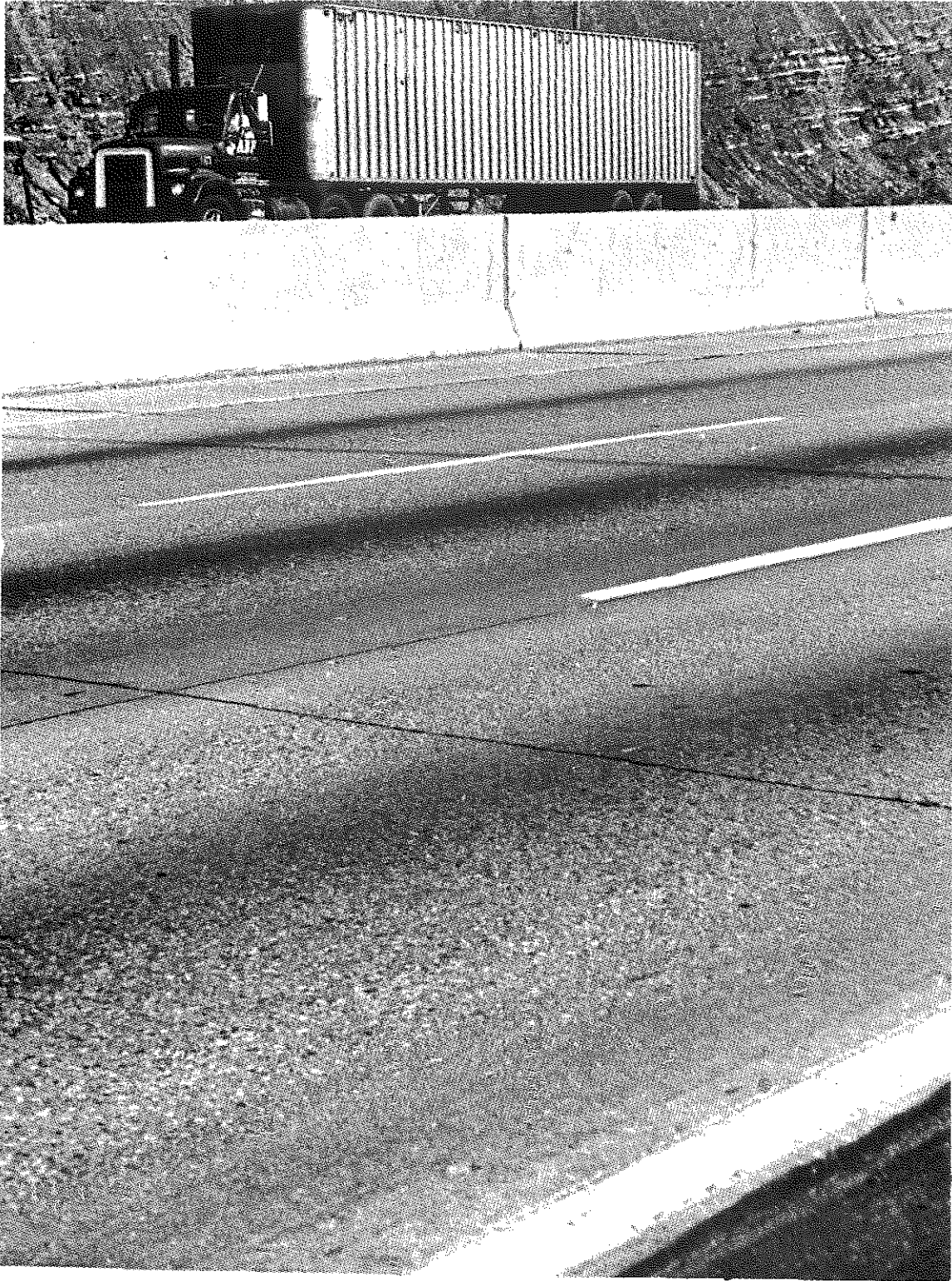
Figure 25. Wear and Rutting, Attributed to Studded Tires.
