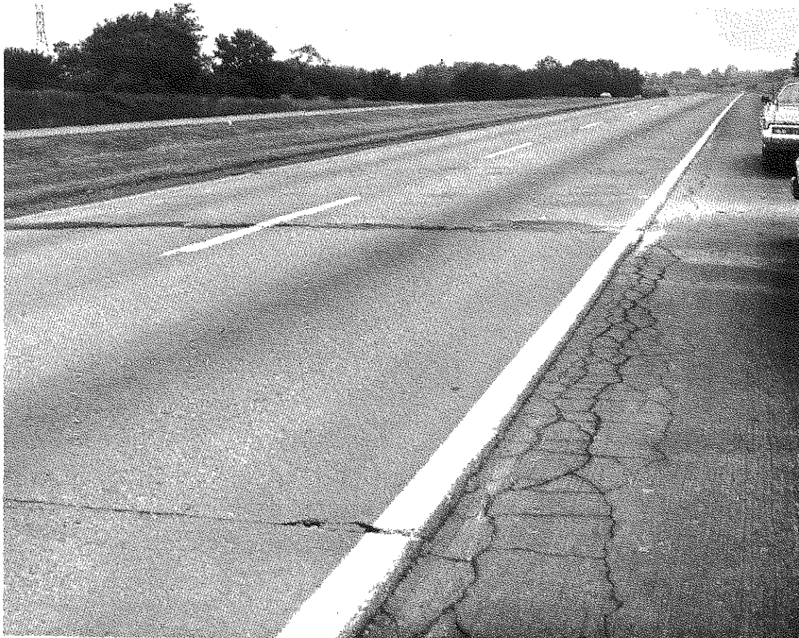
Figure 21. Progressive Deterioration, Arising from Temperature Compression; Sawed, Doweled, Contraction Joints.
