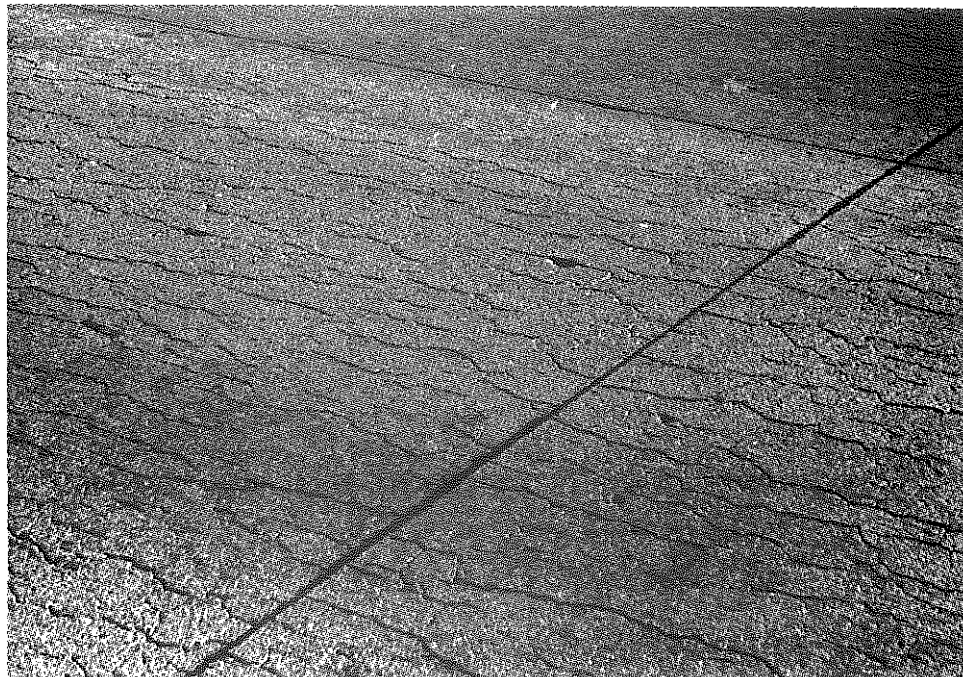
Figure 24. Surface Cracking, Symptomatic of Expansive Aggregate.
