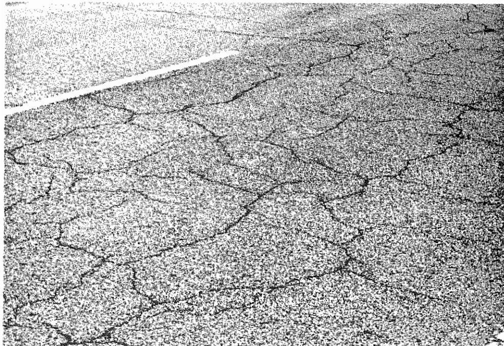
Figure 29. Cracking in an Asphaltic Concrete Surface Course.
