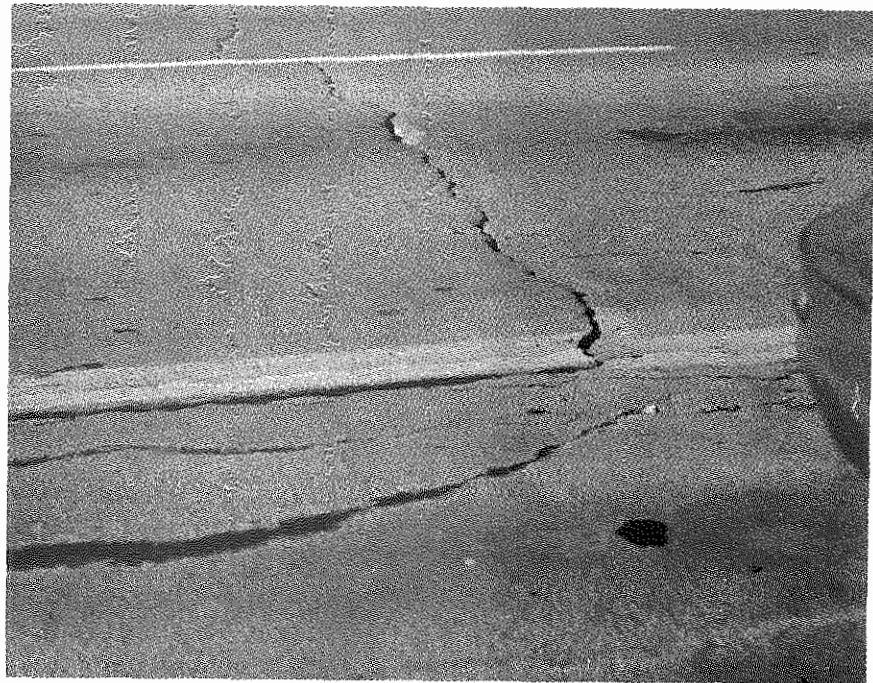
Figure 18. Severe Faulting of a Crack Midway between Non-Functioning Contraction Joints.
