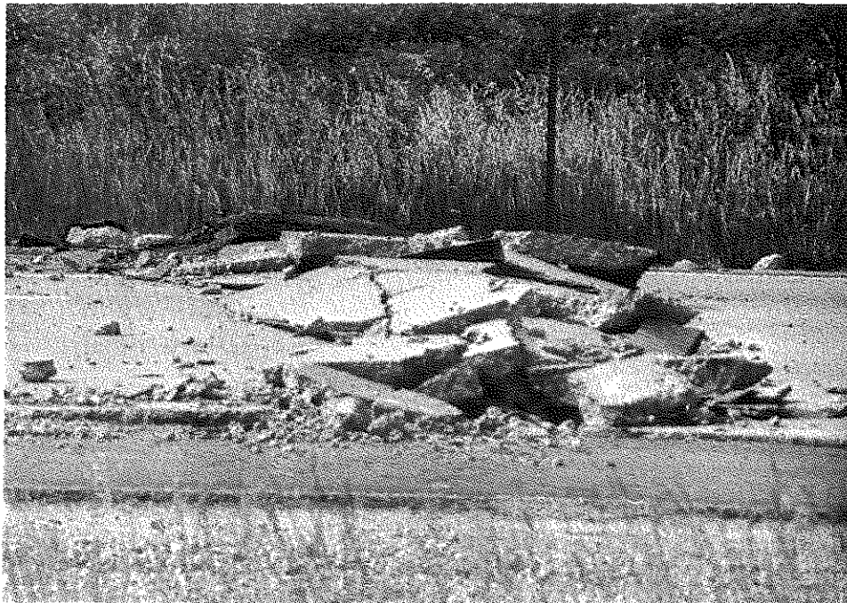
Figure 27. Explosive Upheaval in a CRC-Type Pavement.
