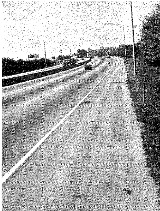
Jefferson County; I 65; North-South Expressway; From Watterson Expressway to Woodbine; Inside Lanes, Median Barrier, and Overlay Added in 1970; Recent Photo.
