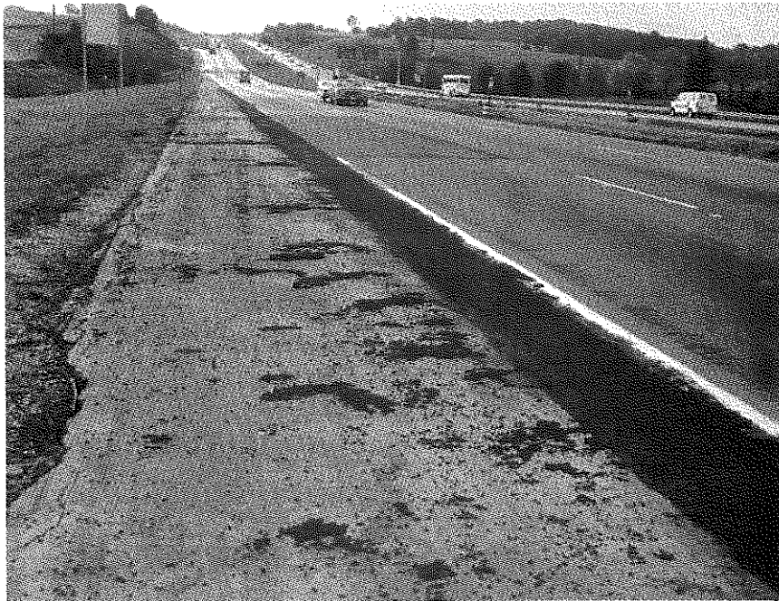
Boone County; I 75; From I 71 to US 42; Shows R-R-R Work in Progress; Lane-wide Patch Covers Area Fragmented after Proof-rolling; Narrow Patch Covers New, Plastic Drain Pipe; Inner Lane and Concrete Barrier Will Be Added.
