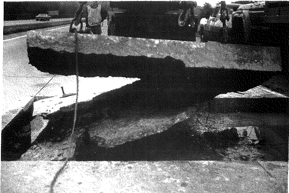
Figure 20. Exposed Joint and Surrounding Concrete; Same Site as Shown in Figure 19.
