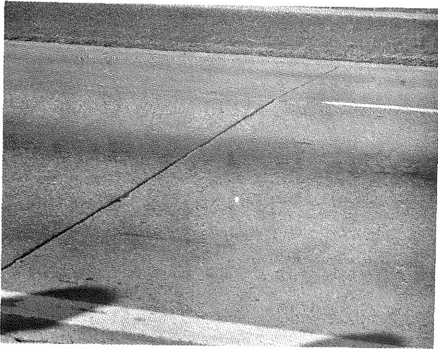
Figure 17. Faulting of a Sawed, Doweled, Contraction Joint; Outer Lane.
