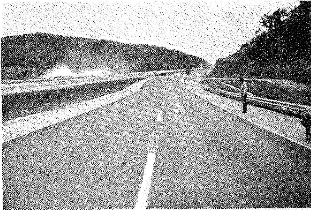
Figure 31. New Asphaltic Concrete Surface Constructed under Traffic; Tendency for Glazing and Apparent Bleeding Shown in Background.
