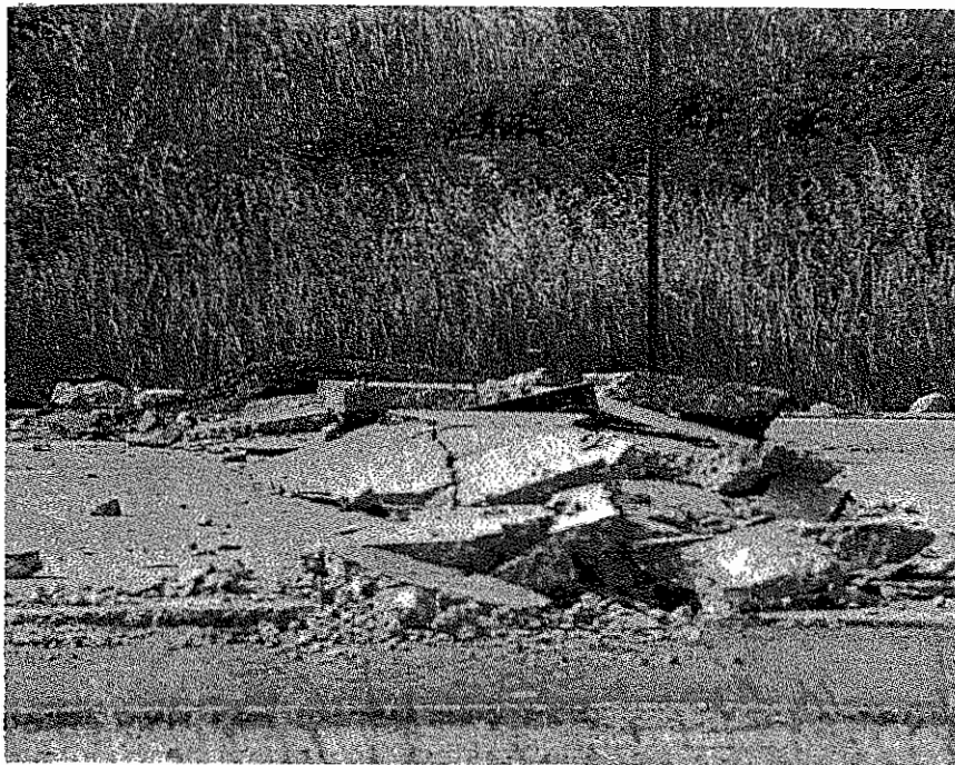
Figure 15. Different View of Failure Shown in Figure 14 (Madison Courier; May 21, 1977).
