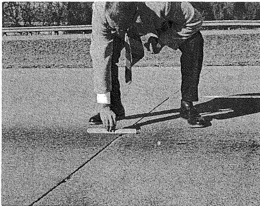
Figure 9. Contraction Joint which Is also Faulted Slightly in One Lane.
