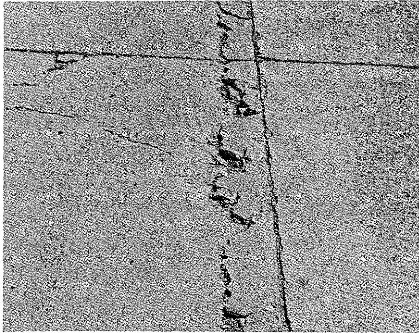
Figure 12. Severe D-Cracking; Airport Apron.
