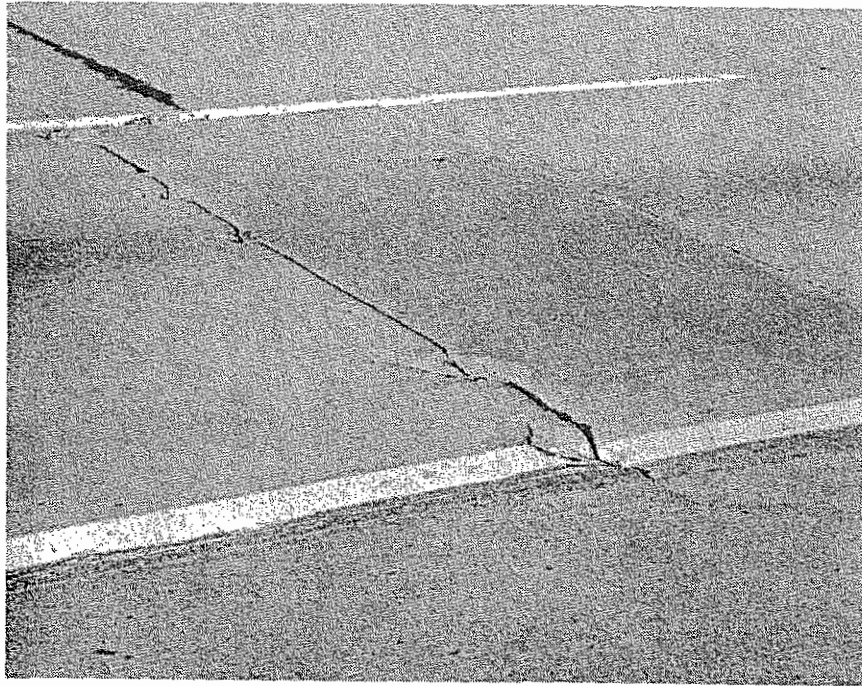
Figure 10. Upthrusting at a Full-Depth, Inverted-T Patch.
