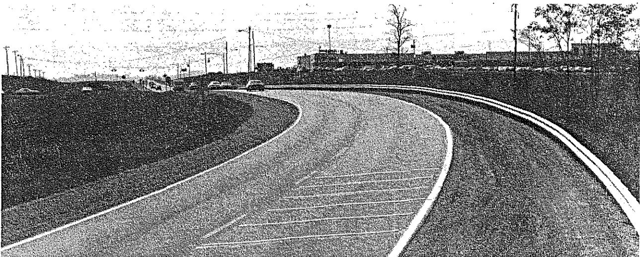
Figure 8. Reflective tape on southbound approach at the intersection of US 127 and US 150 (two layers of Stamark tape).
