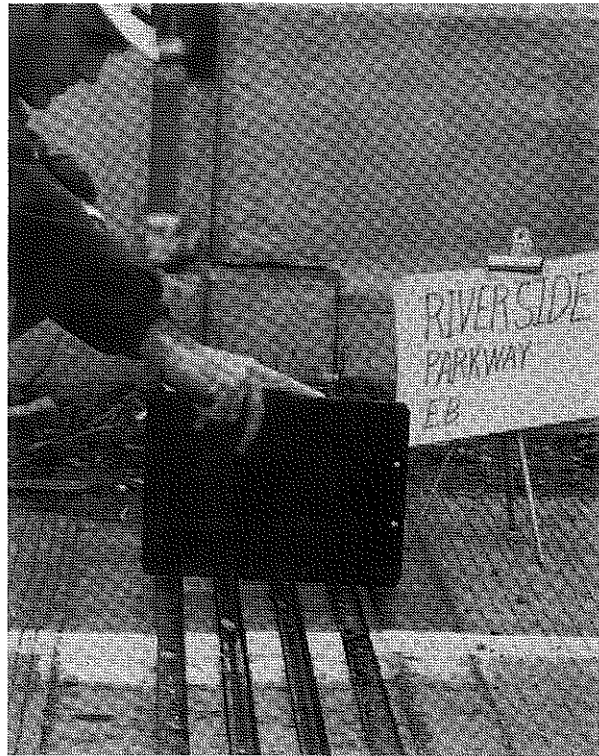
Figure A26. Wabo-Maurer D1040; note vertical misalign- ment across the joint.
