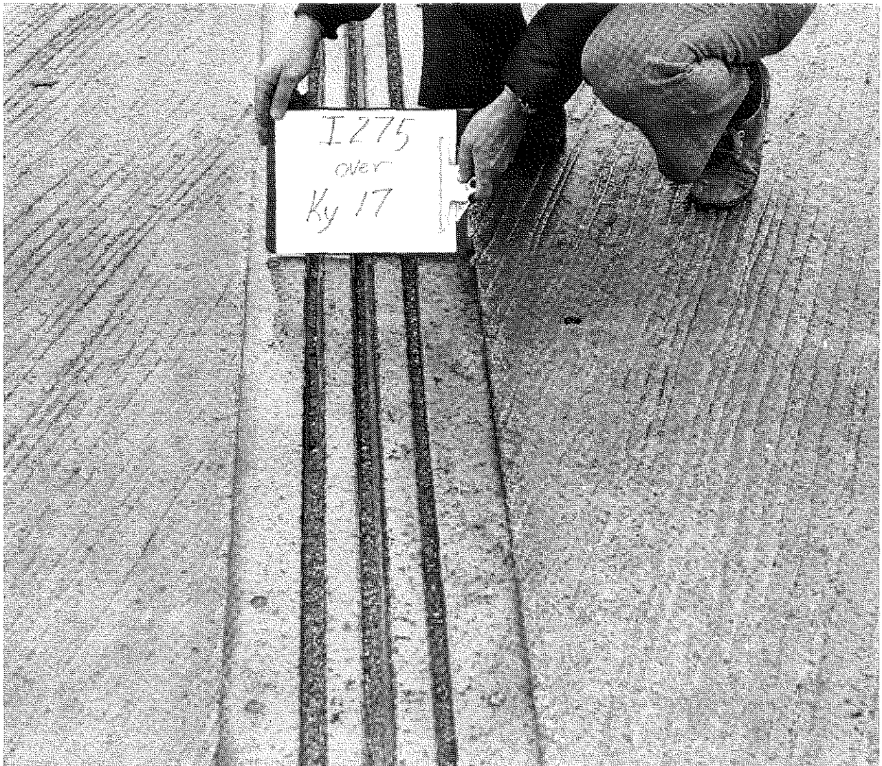
Figure A7. Acme, Acma Modular II 3M600; note debris above seals.
