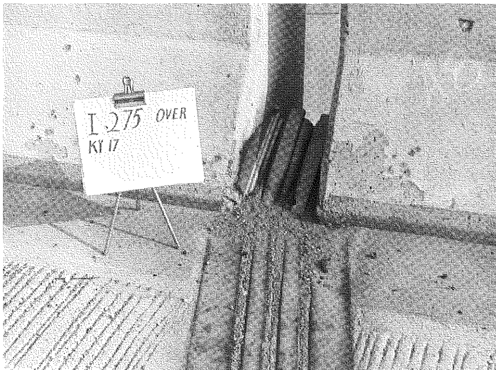
Figure A8. Acme, Acma Modular II 3M600; note debris in gutter area.
