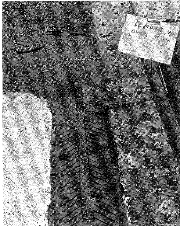
Figure A16. Fel Span T20; note edge sealant and deterioration of the hole plugs.
