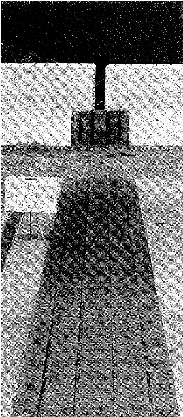
Figure A21. Transflex 400A; note accumulation of debris and initial deterioration of the hole plugs.
