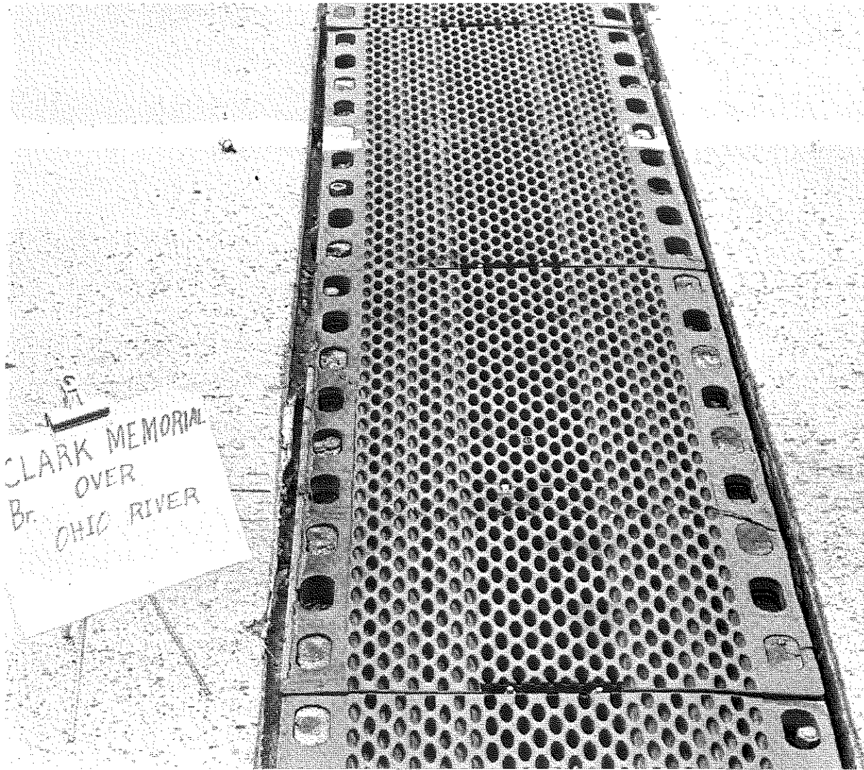
Figure A34. Transflex 400; no edge sealant, no hole plugs, misalignment of the abutted sections, open grid system collects debris.
