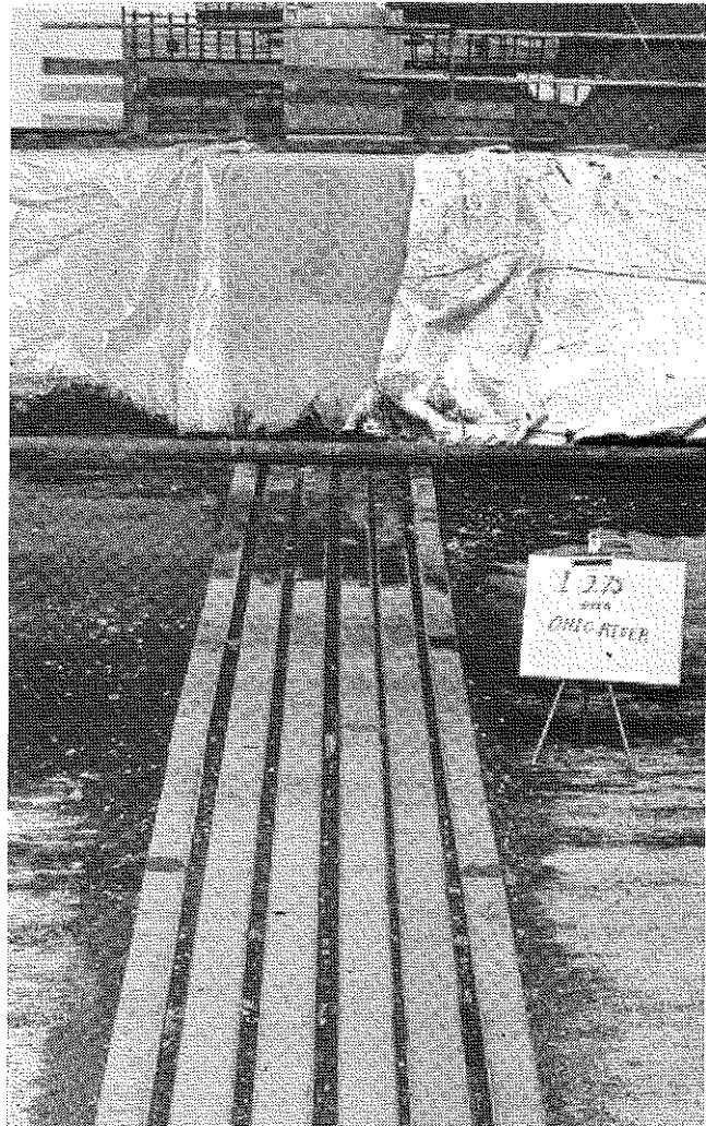
Figure A6. Wabo-Maurer D1300; note uneven compression of seals.
