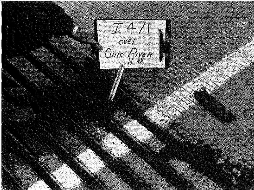
Figure A9. Wabo-Maurer D1560; note cavity above seal and pavement surface and accumulation of debris.
