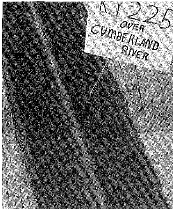
Figure A25. Fel Span T40; note deterioration of the hole plugs.
