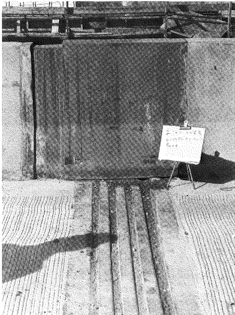
Figure A3. Acme Beta B1300; joint in excellent condition; note debris above neoprene seals.
