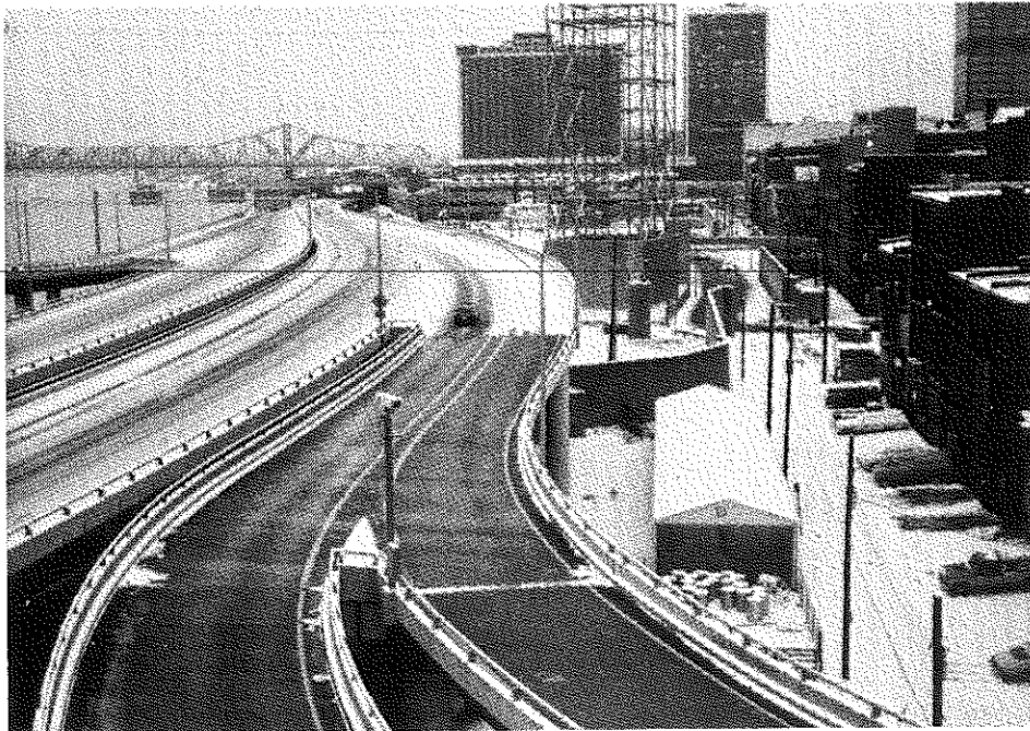
Figure 13. Inoperative Heating Cable (left curb); January 13, 1982.
