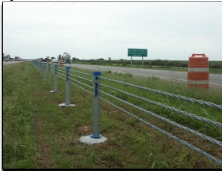
Figure 1: Four Strand, Cable Median Barrier
