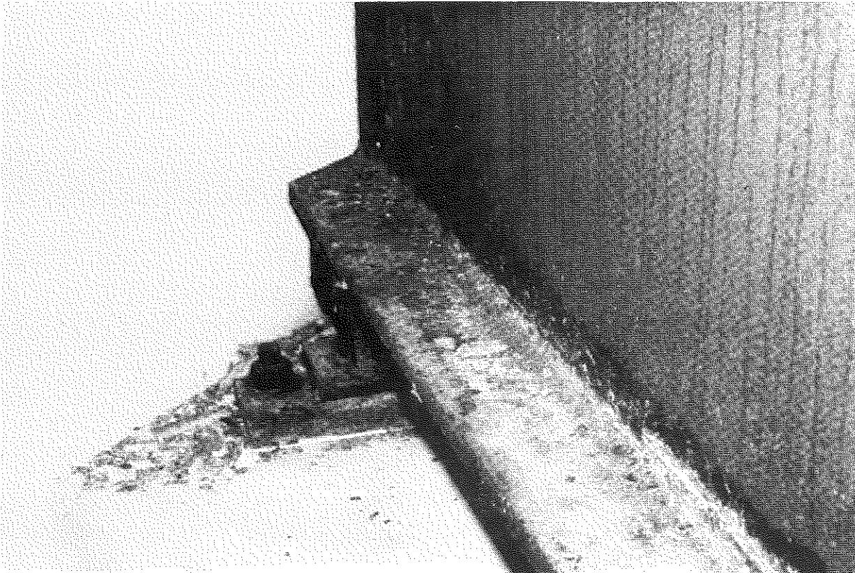
Figure 13. Abnormal Corrosion on Interior Girder at East End of KY-1893 Bridge.
