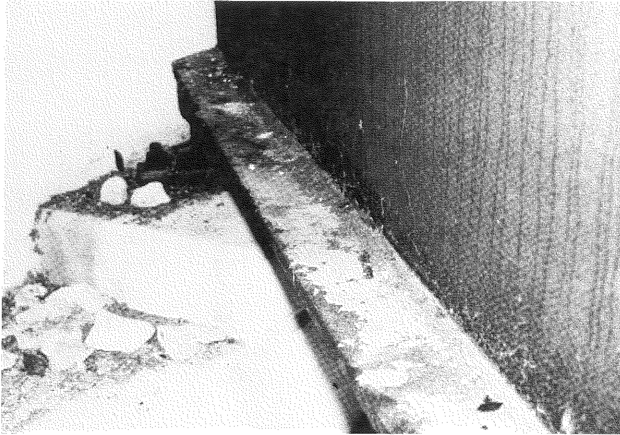
Figure 14. Abnormal Corrosion on Interior Girder at West End of KY-1893 Bridge.
