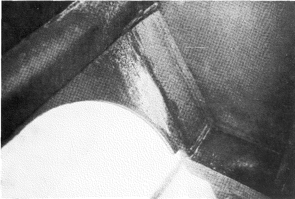
Figure 9. Alloy Segregation Spot on the Equestrian Bridge Showing No Visible Corrosion.
