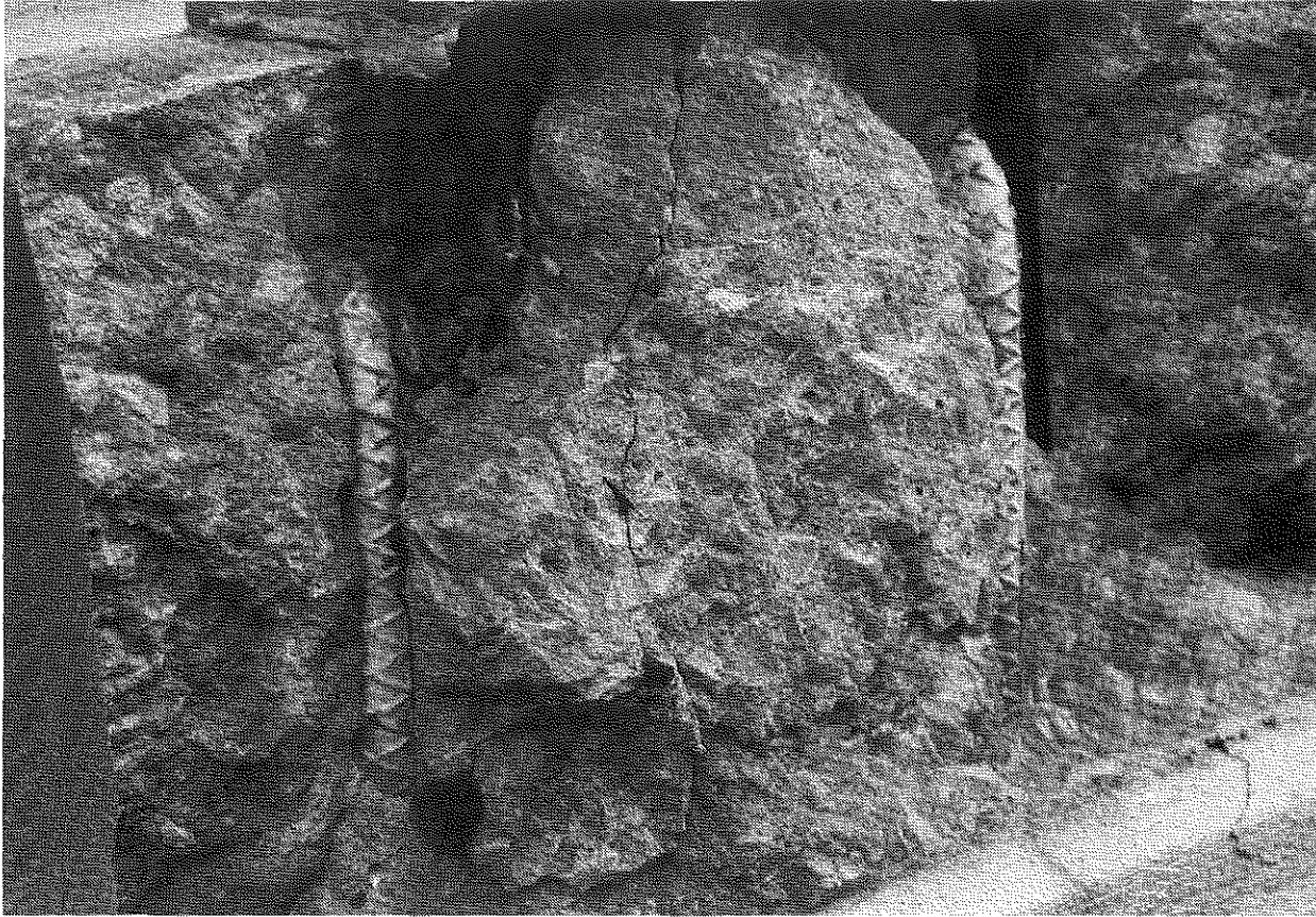
Figure 5. Broken Epoxy and Rust on Exposed Reinforcing Steel, US-45 Bridge at Brookport, IL (1982).
