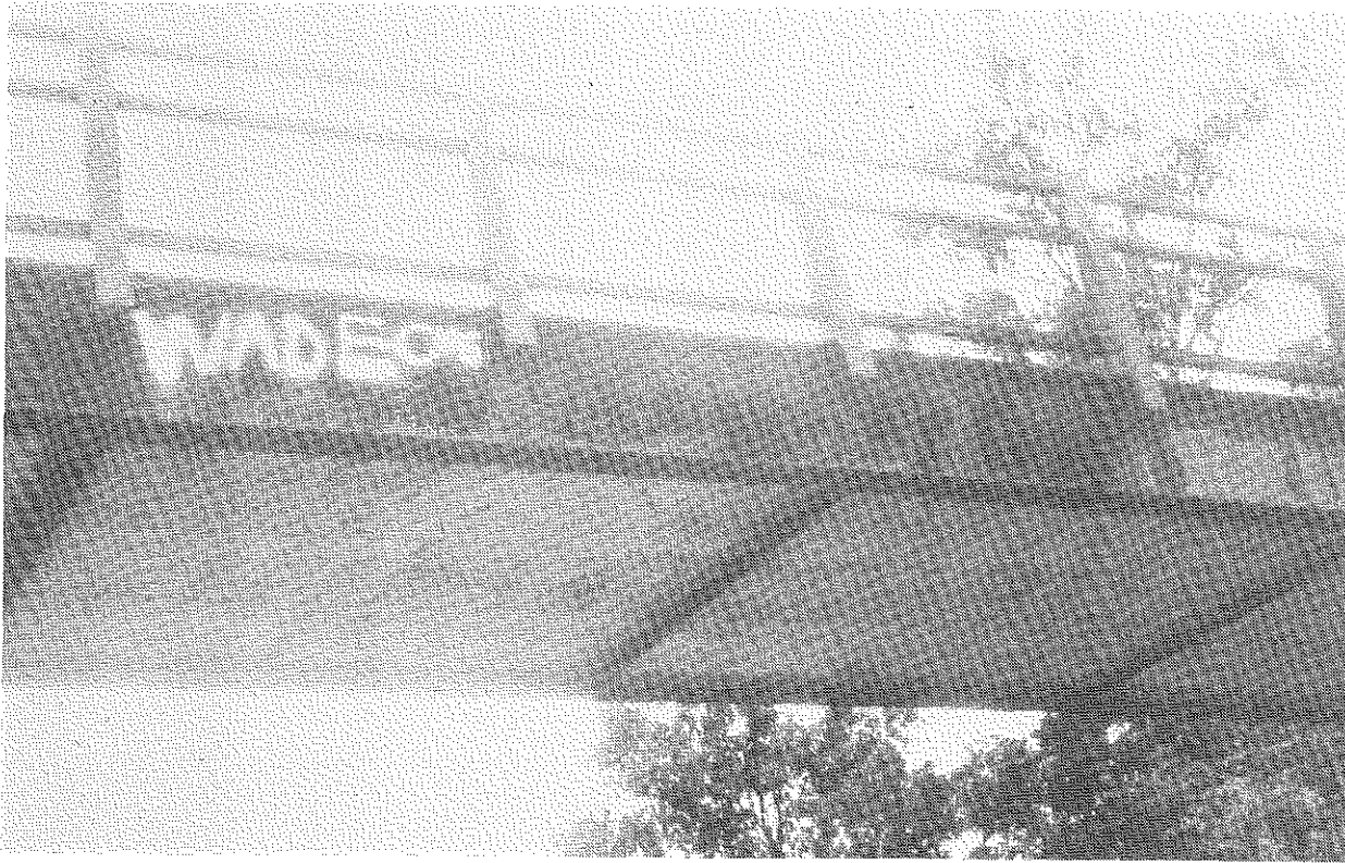
Figure 18. Graffiti (Spray Paint) on Girder of the Equestrian Bridge at Louisville.
