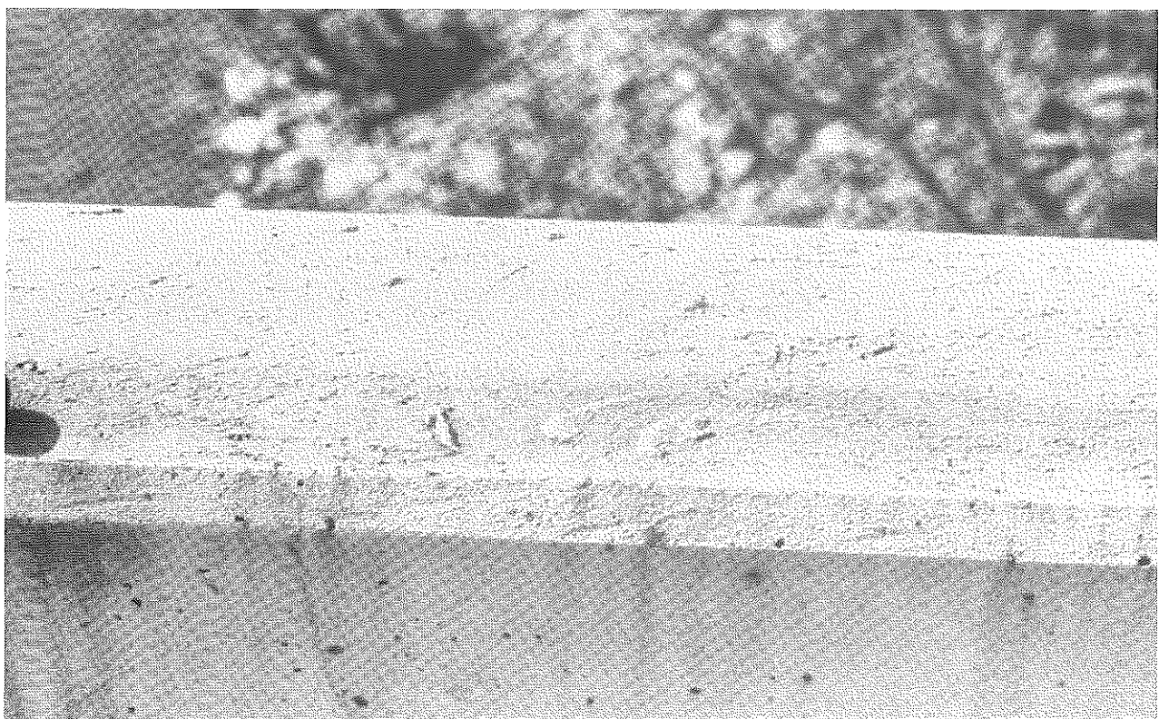
Figure 36. Uneven Masonry Coating on KY-35 Bridge.
