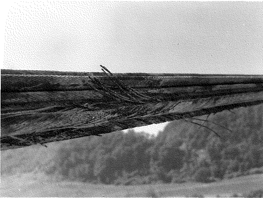
Figure 11. Portion of a Cable previously Covered by a Cable Band (Stage 4 Corrosion Damage) (1979).
