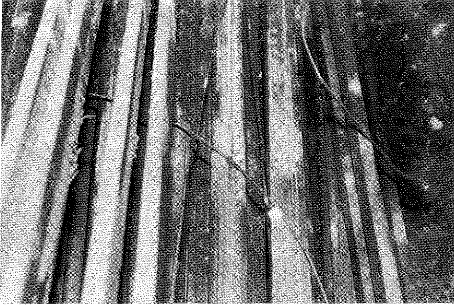
Figure 20. Broken Wires and Water Leakage Stains in the Upstream Kentucky Anchorage of the Ohio Bridge (1980).
