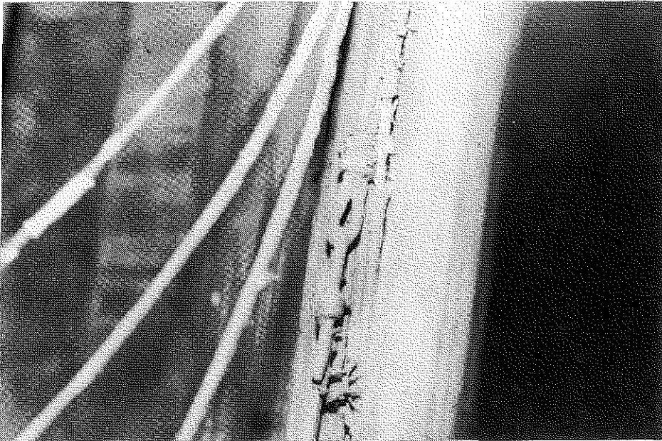
Figure 21. Repair Splice on Wires in Upstream Kentucky Anchorage of the Ohio Bridge (1980).
