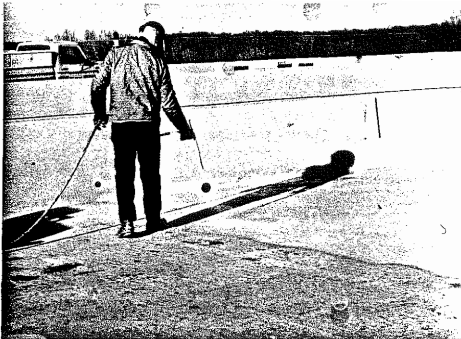
Figure 4. Sealing of the I-24 Bridge over the Cumberland River with a Concrete Curing Compound (1980).
