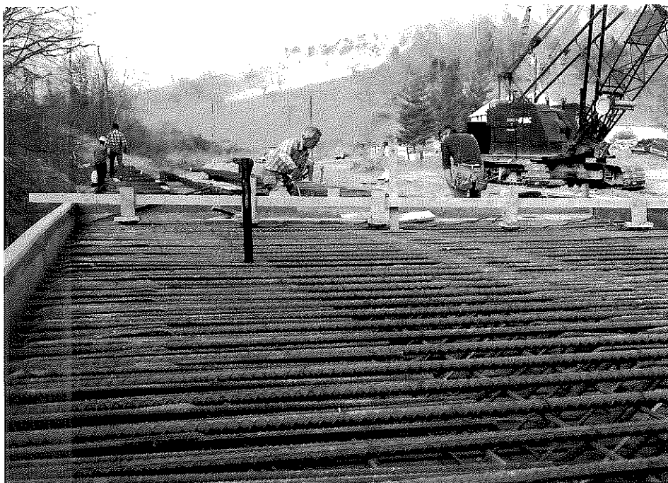
Figure 25. Photo of Earth Pressure Meters Prior to Placement of Top Slab Concrete.
