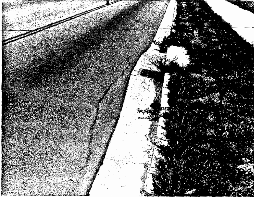
Figure 5. Shrinkage Cracking around Concrete Inlet Drain
