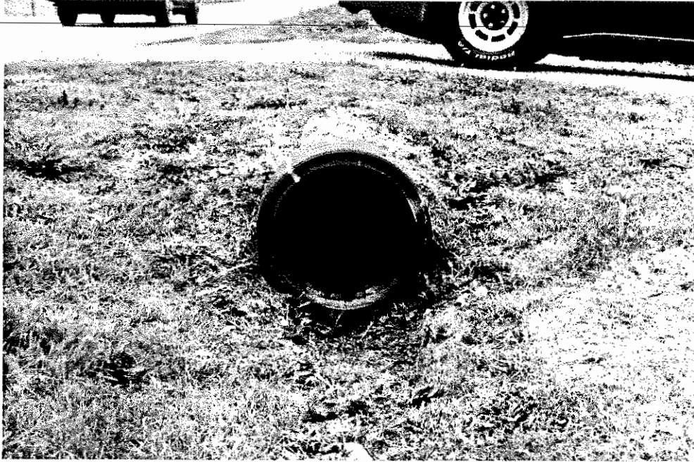
Figure 1. Grass Lined Channel Prevents Erosion; KY 130, Union County.
