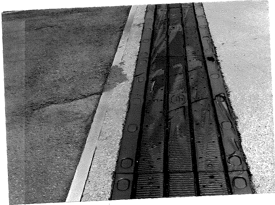
Figure 3. A Transflex 650 Joint Exhibiting Surface Abrasions and Gouges.
