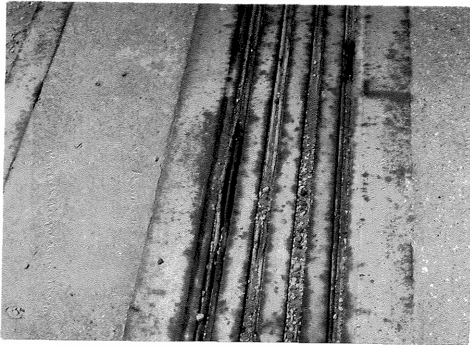
Figure 1. Loose Module Seal on Wabo-Maurer D1040 Joint on the US 27 Bridge over the Kentucky River at Camp Nelson.
