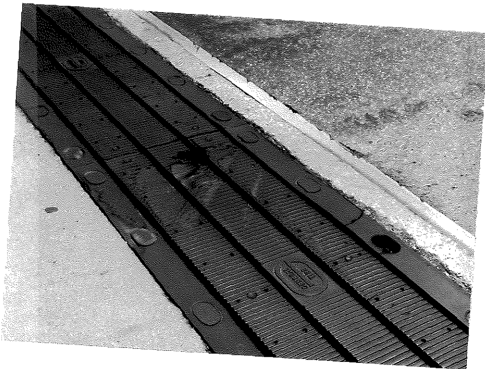
Figure 4. Missing Stud Cover on Transflex 650 Joint on the US 421 Bridge over the Cumberland River.
