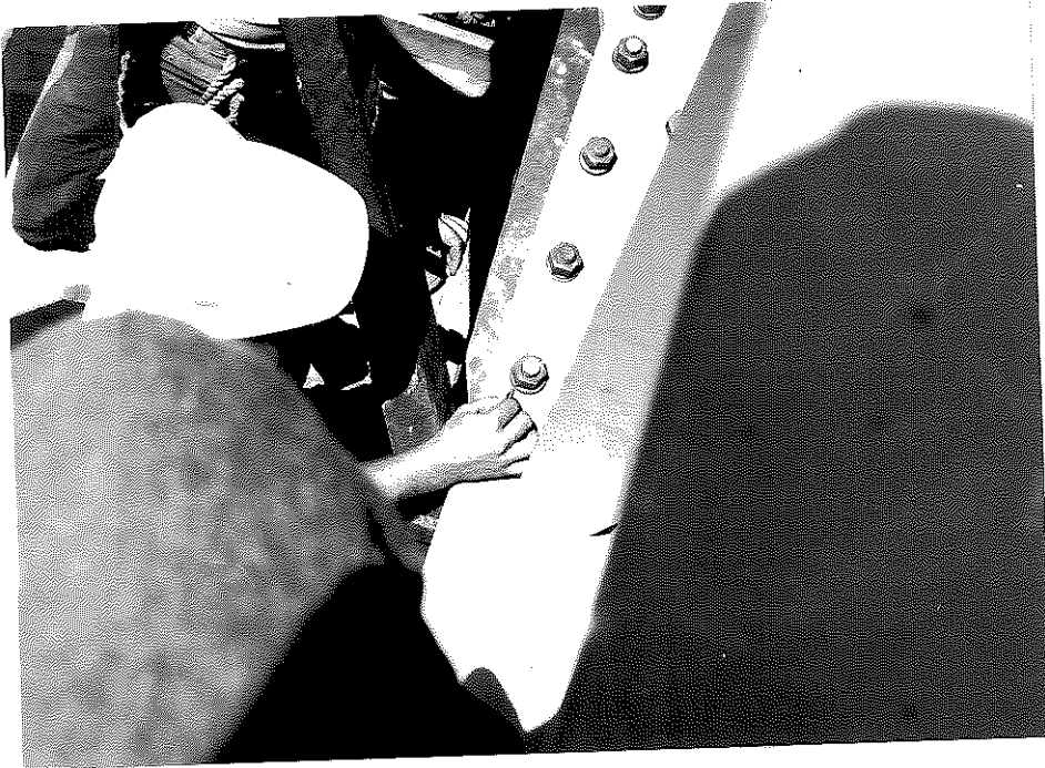
Figure 4. A State Inspector Checking the Gap of a LIW Used on a Flange Splice.
