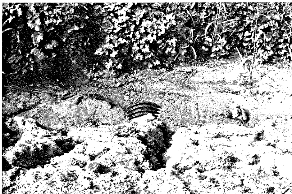
Photo 3. Silted pipe in Owensboro.
