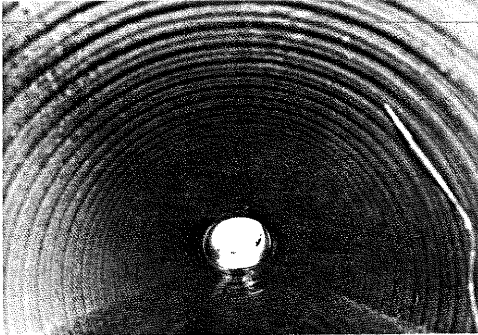
Photo 10. Pipe deflection at Station 167+50 (18-inch pipe).
