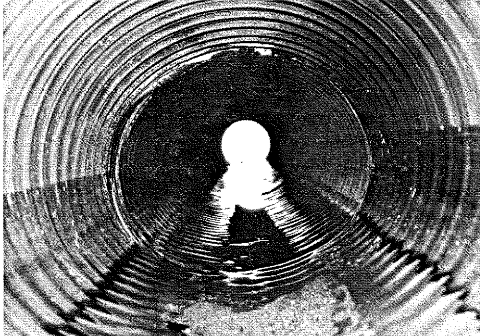
Photo 8. Compression in a 24-inch entrance pipe at Station 174+00.
