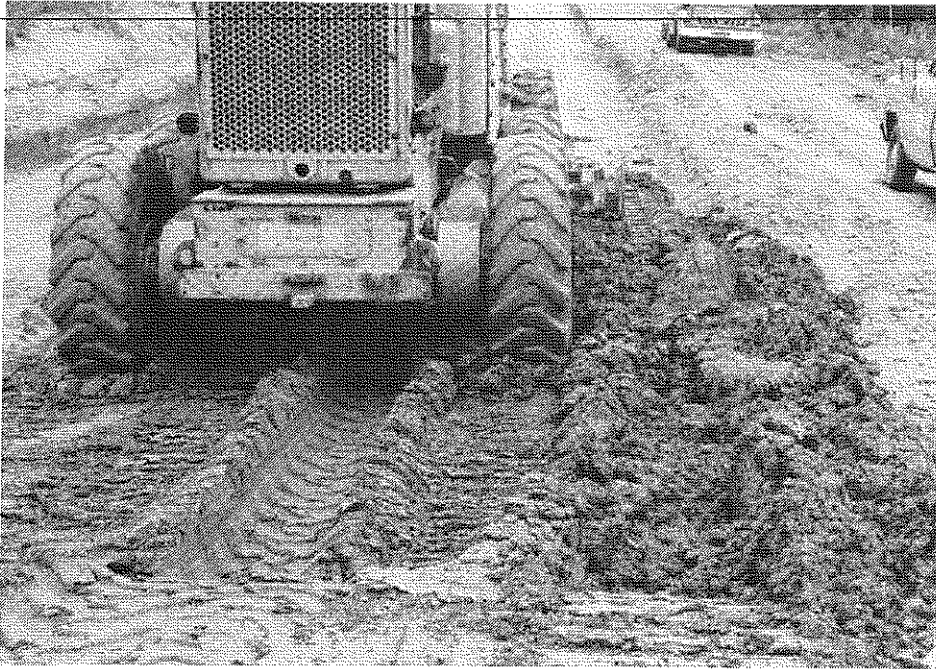
Figure 12. A road grader was used to spread the first two loads of the AFBC stabilized pond ash subbase mixture.
