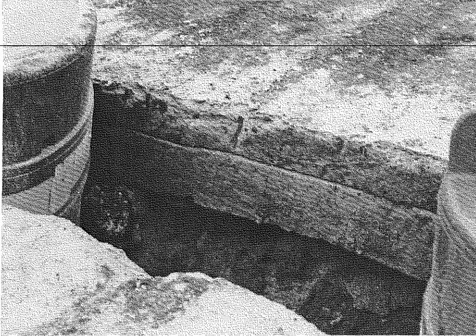
Figure 28. Differential expansion between the first and second lifts of the AFBC stabilized pond ash mixture was observed in the trenched areas.
