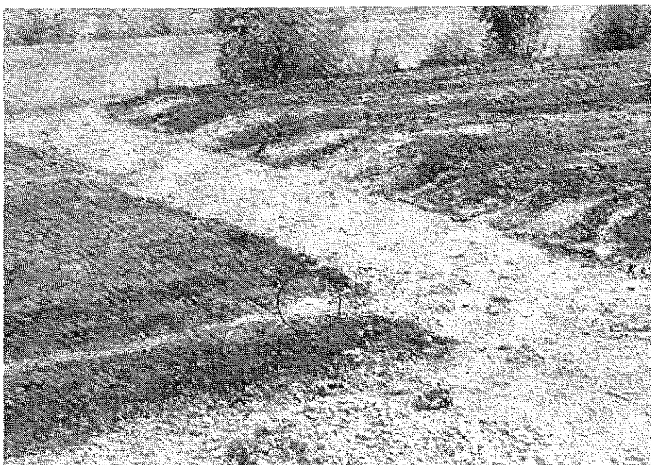
Figure 25. Survey pins were grouted into the AFBC concrete base layer. Expansion of the base layer is evidenced by the wave formed on the surface of the subgrade.
