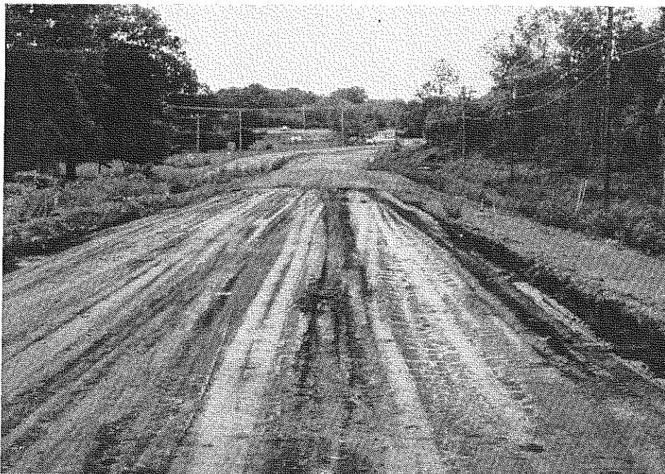
Figure 15. Deep ruts formed in the plastic subbase mixture when the curing seal was placed too soon after completing compaction.
