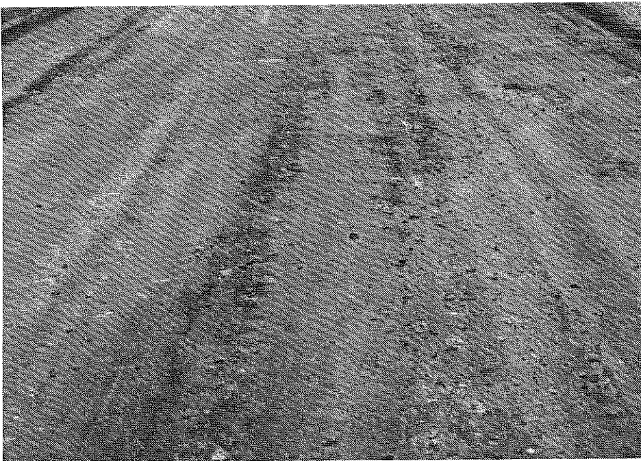
Figure 19. Longitudinal centerline cracking and wheel-track rutting in the AFBC concrete base section.
