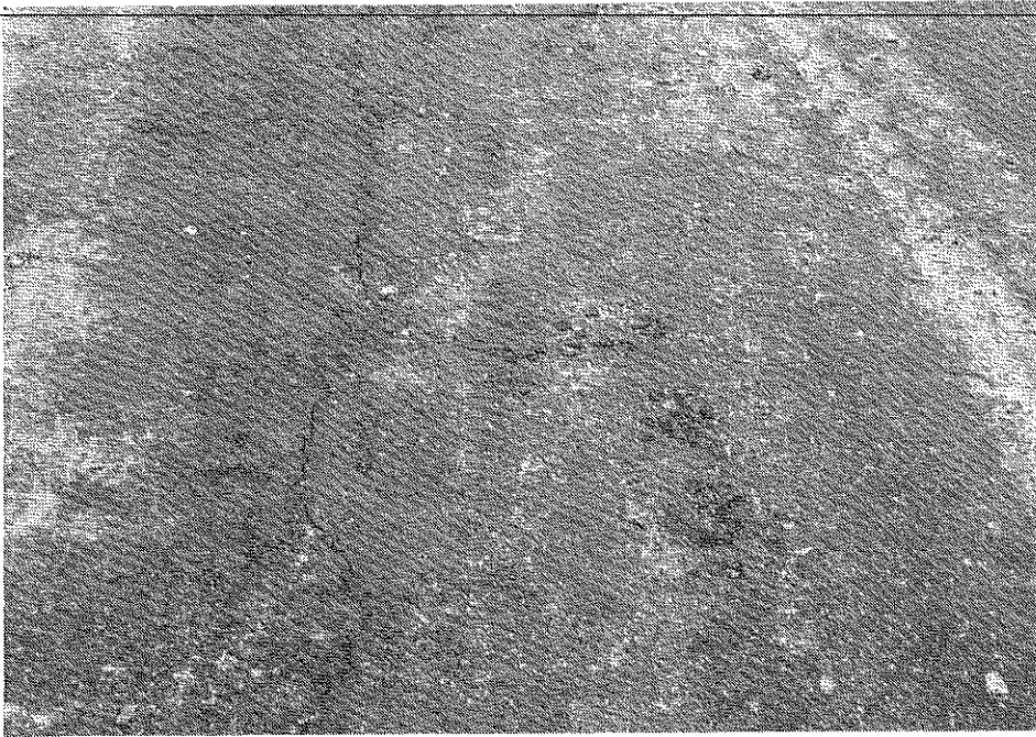
Figure 20. Longitudinal and transverse cracking observed in the AFBC concrete base section.
