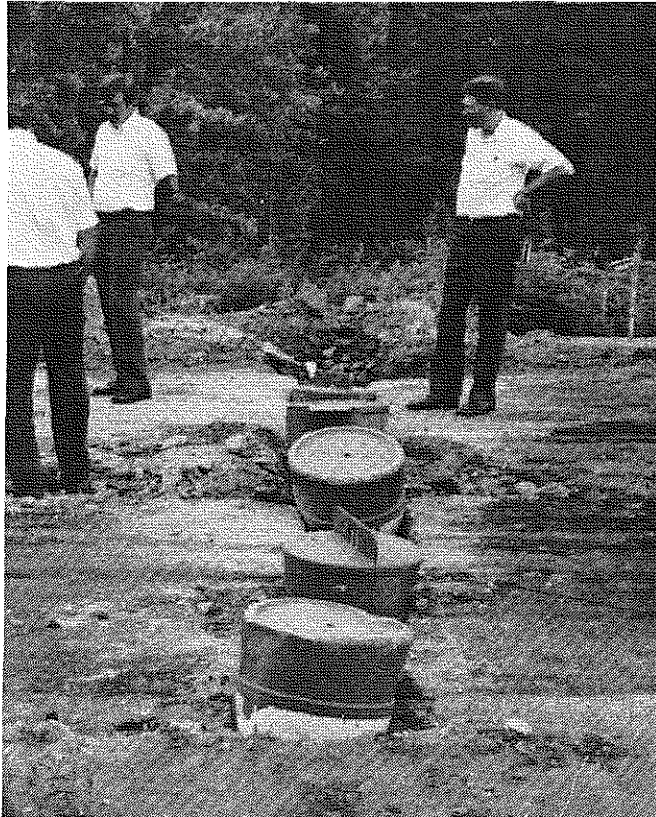
Figure 27. Expansion of the AFBC stabilized pond ash mixture crushed the orange safety barrels that were placed in the trench.
