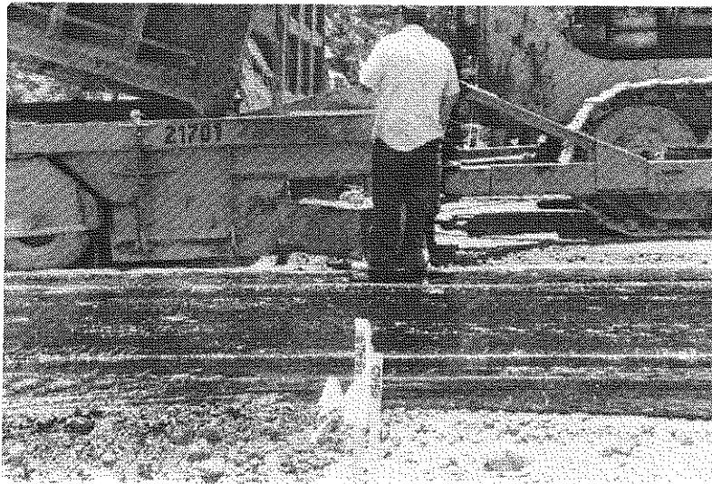
Figure 14. Placement operations continued in the eastbound lane after the curing membrane had been applied in the westbound lane.
