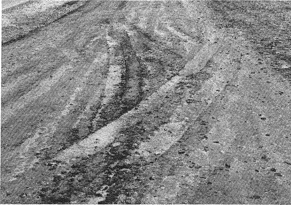
Figure 11. The plastic AFBC concrete base was easily rutted when the curing seal was applied.
