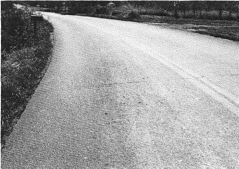
Figure 13. Reflective Cracking was Evident in Both Experimental and Control Sections.
