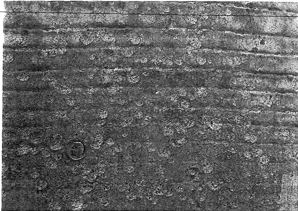
Figure 6. Numerous microcracks were observed on the experimental PBC concrete bridge deck during the initial inspection.
