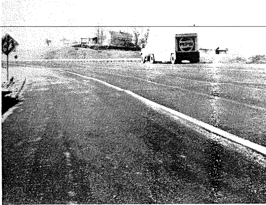
Figure 24. View of humps on pavement surface near Station 560+00.
