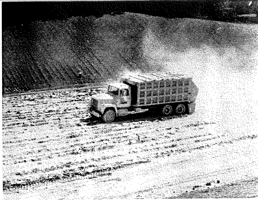
Figure 22. The prepared subgrade was ripped prior to distributing the multicone kiln dust with the spreader truck.
