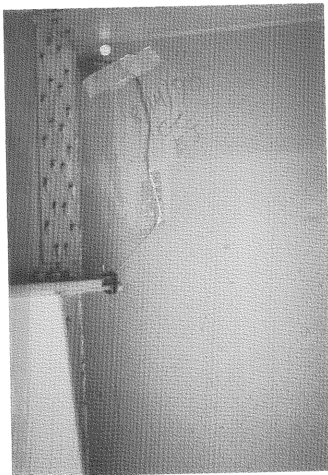
Figure 4. Strain Gage Located Adjacent to Floorbeam on KY 80 over Russell Fork of Big Sandy River and CSX R.R., Pike Co. (B-137).
