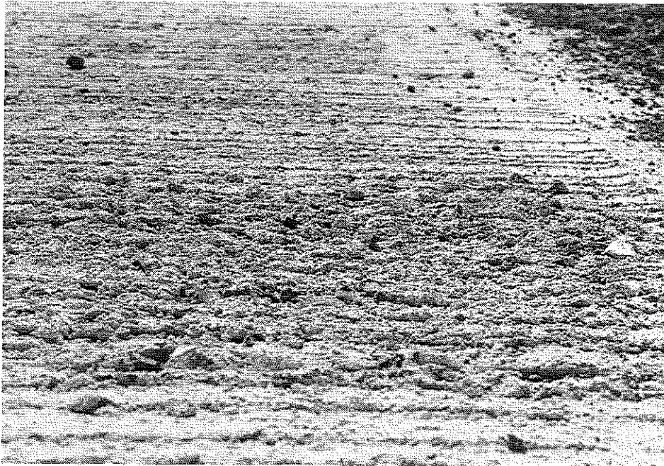
Figure 2. The surface finish of the experimental deck was unsatisfactory.
