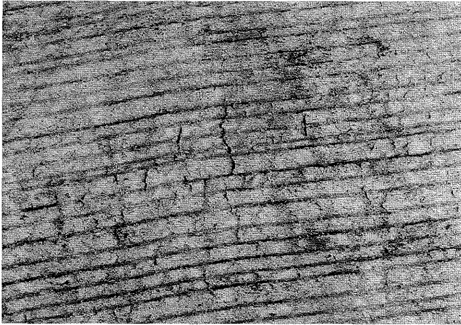
Figure 3. Surface cracking was apparent after the curing blankets were removed.
