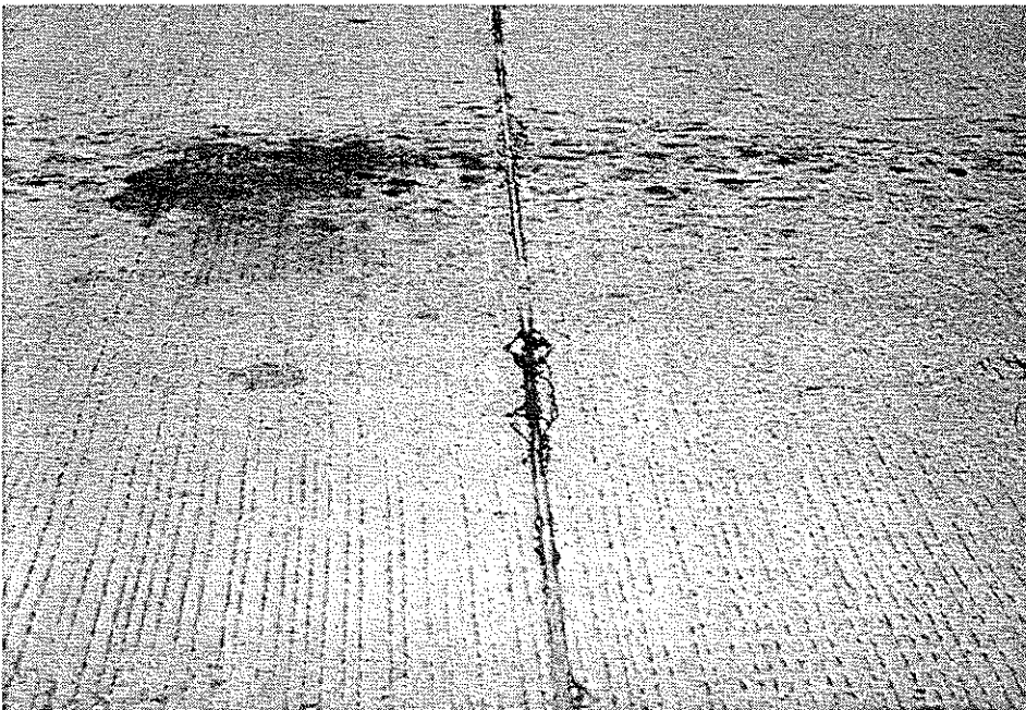
Figure 2. Typical distressed pavement joint at intersection of US 31E and US 68/KY 80.
