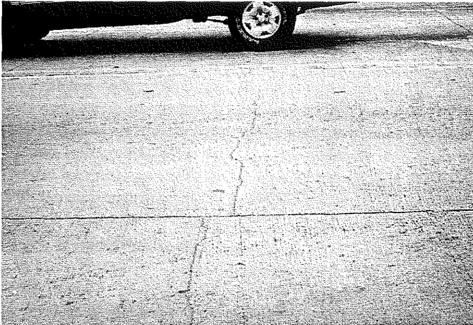
Figure 1. Typical mid-slab crack of PCC pavement at intersection of US 31E and US 68/80
