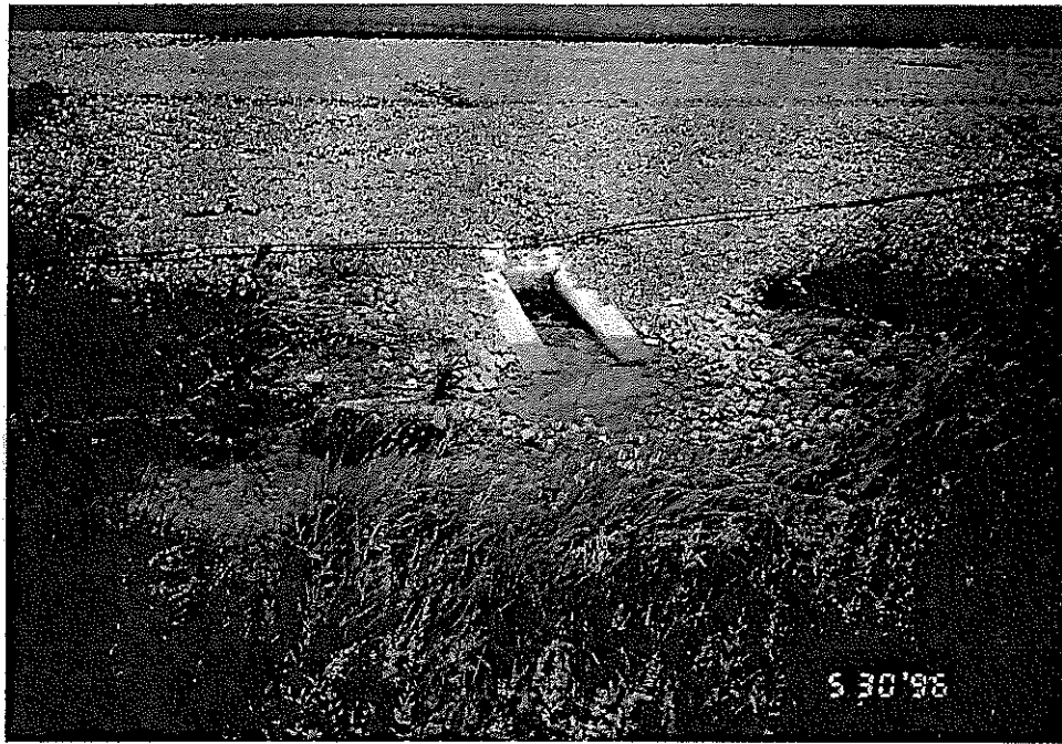
FIGURE 9. HEADWALL TOO LOW IN DITCH LINE, PARTIALLY UNDER WATER.
