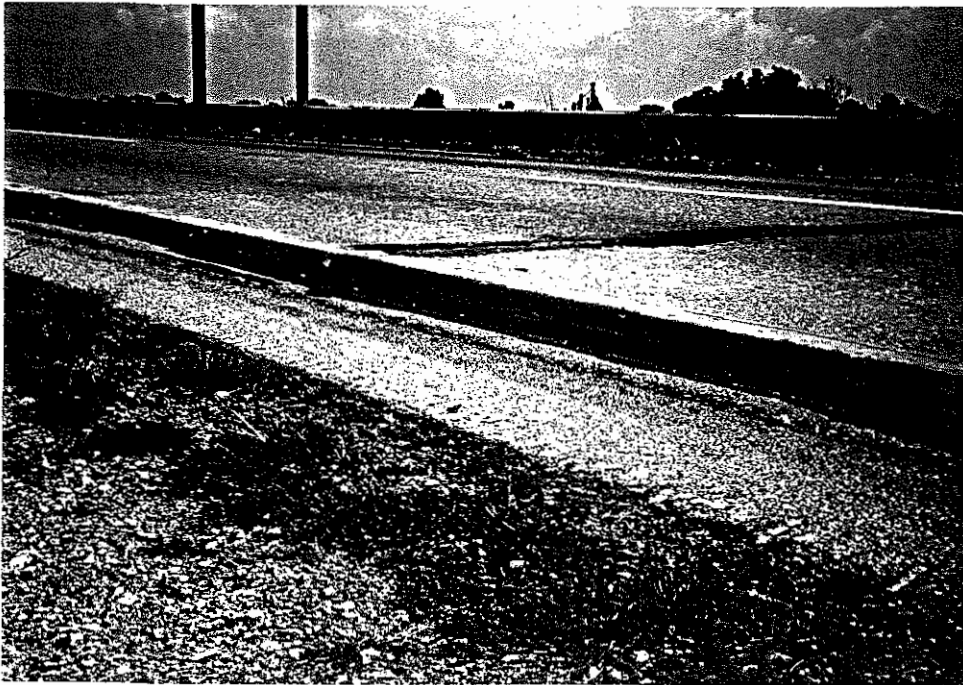
Figure 17. Settlement in edge drain trench due to traffic being forced onto the shoulder.
