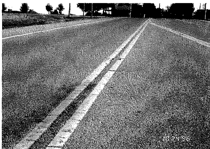
Figure 13. Bleeding observed at Station 183+75.
