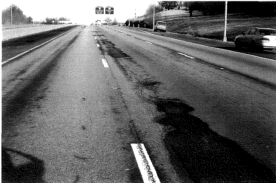
Figure 1. Delamination and Potholes on I-75.
