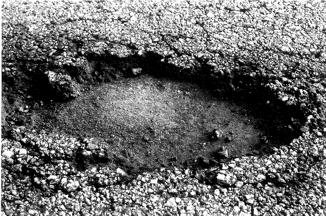
Figure 2. Showing Debonding of the Two Surface Lifts
