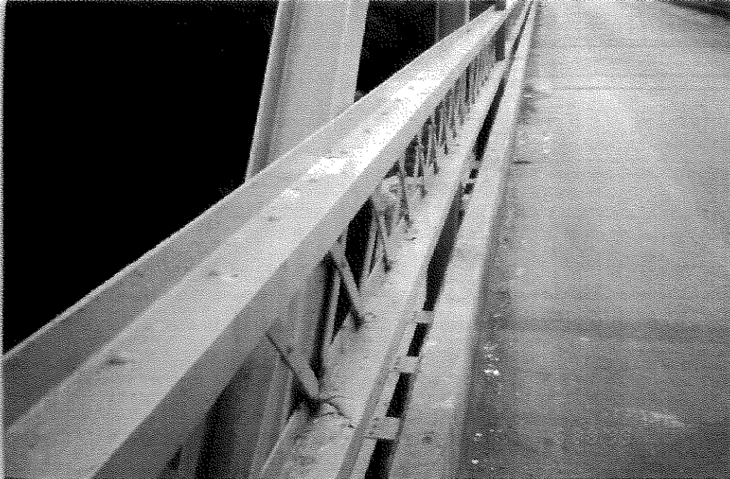
FIGURE 55. KY 22 BRIDGE GUARDRAIL SHOWING DISBONDING ON HORIZONTAL SURFACE OF TOP RAIL.
