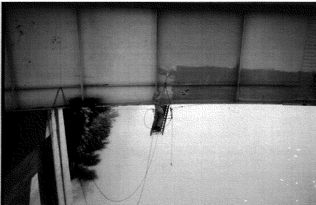
FIGURE 6. TRUSS ON THE KY-22 BRIDGE SHOWING EXTENSIVE REMOVAL OF THE EXISTING PAINT BY PRESSURE WASHING. PAINTER IS USING A MITT TO APPLY THE SPOT PRIMER.
