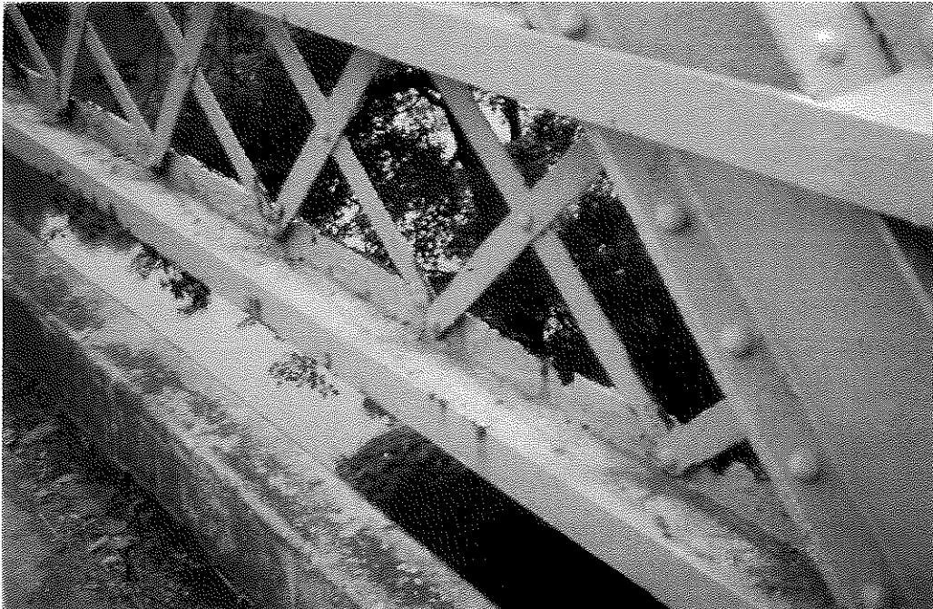
FIGURE 54. KY 22 BRIDGE GUARDRAIL SHOWING EXTENSIVE COATING FAILURE AT EDGES OF LACING BARS.
