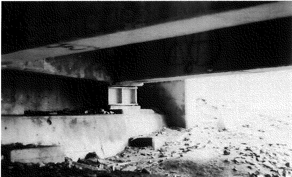
FIGURE 34. I-71 CONCRETE OVERPASS BRIDGE SHOWING STEEL BEARING CORROSION (1997).
