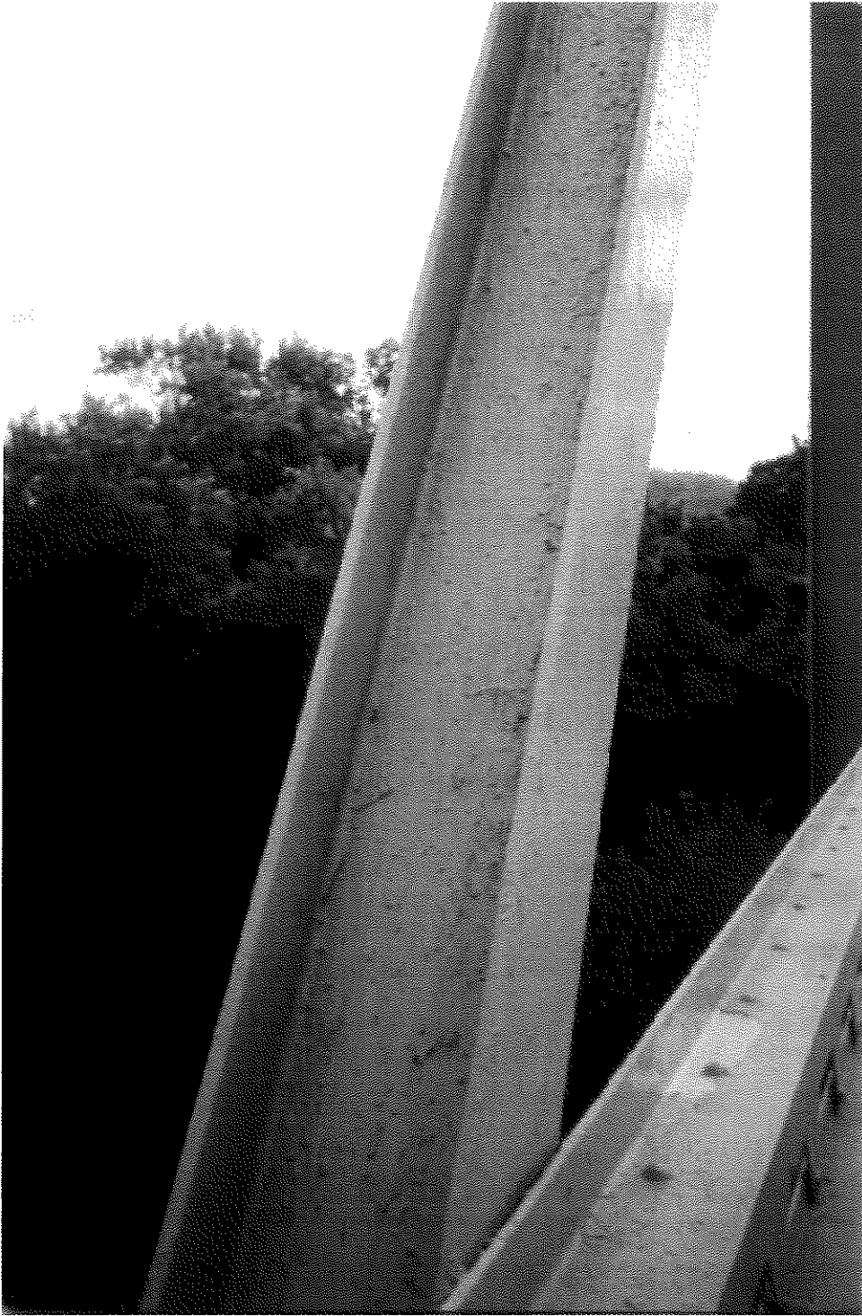
FIGURE 57. KY 22 BRIDGE DIAGONAL SHOWING PAINT RUNS AND DIRT BUILD-UP.
