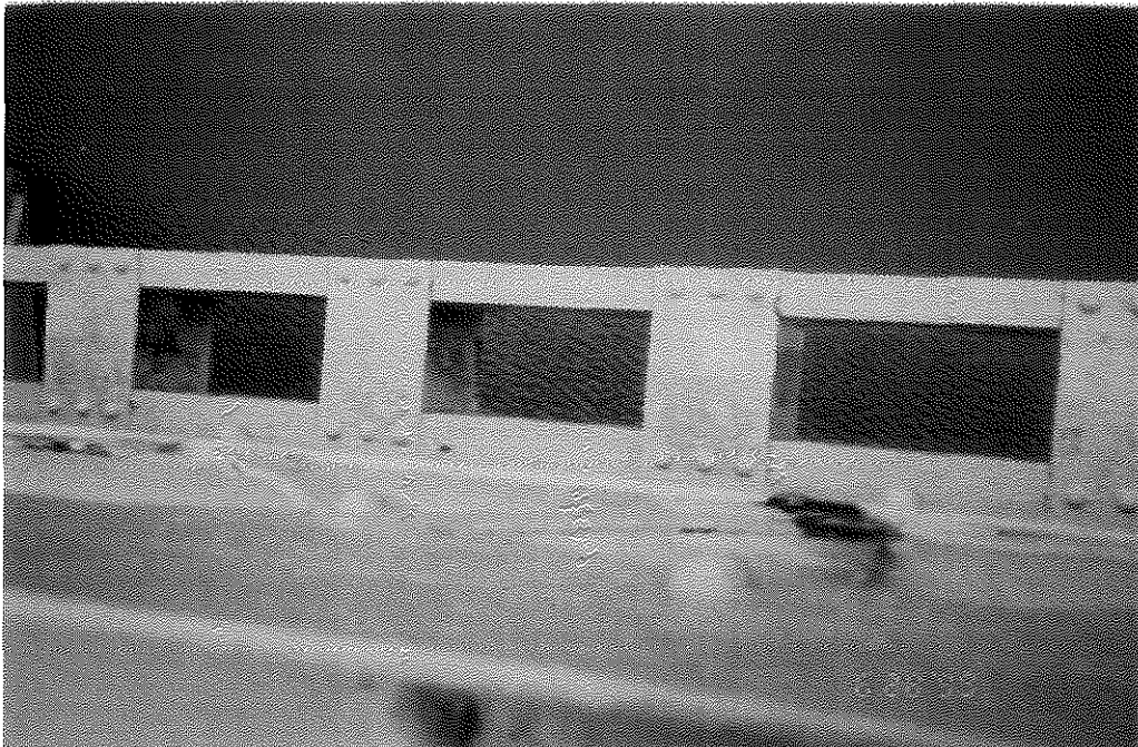
FIGURE 50. BATTEN PLATES ON DOWNSTREAM LOWER CHORD OF KY 22 BRIDGE SHOWING PAINT IN GOOD CONDITION.
