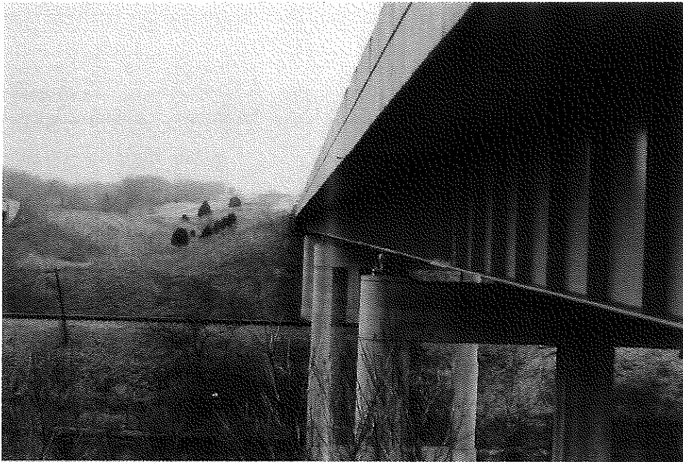
FIGURE 37. I-71 STEEL MAINLINE BRIDGE OVER SULPHUR CREEK AND THE CSX RAILROAD SHOWING PAINT IN GOOD CONDITION (1997).
