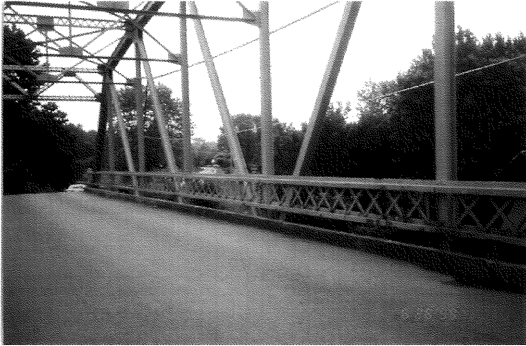
FIGURE 53. KY 22 BRIDGE GUARDRAIL SHOWING EXTENSIVE COATING FAILURE.
