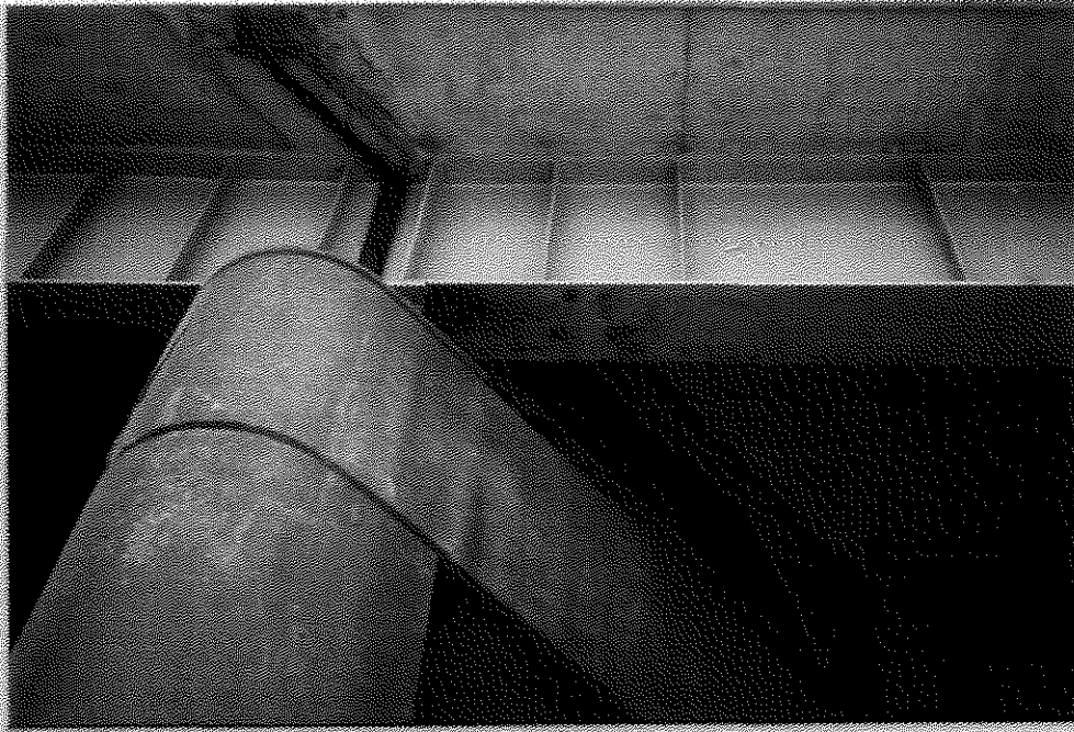
FIGURE 41. KY 146 OVERPASS BRIDGE OVER I-71 SHOWING CORROSION ON LOWER FLANGE UNDER DECK JOINT (1999).
