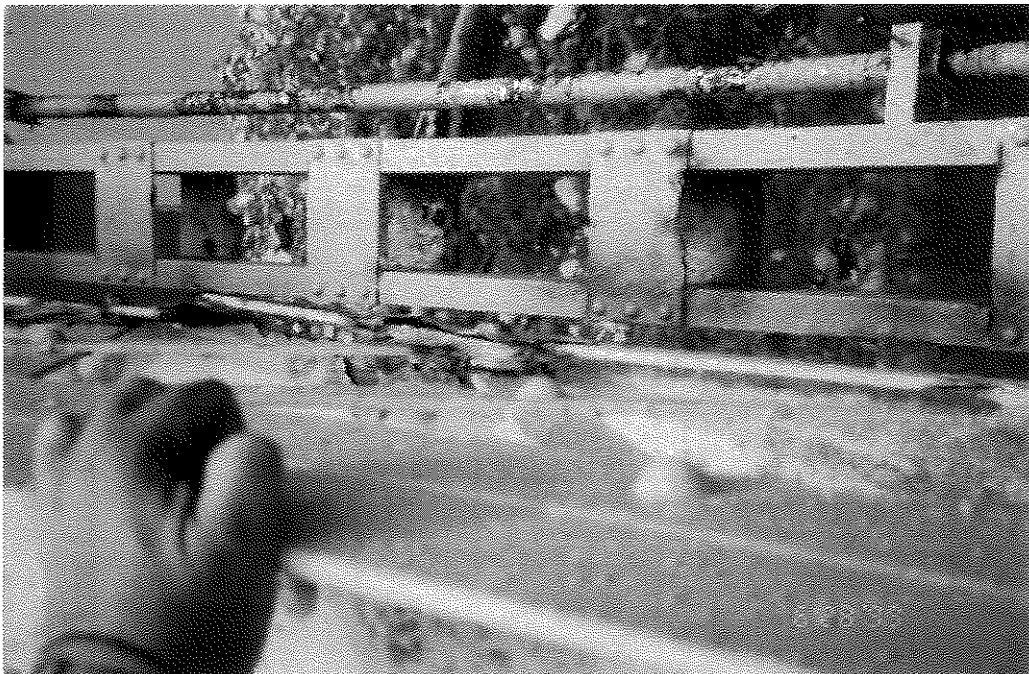
FIGURE 52. BATTEN PLATES ON UPSTREAM LOWER CHORD OF KY 22 BRIDGE SHOWING COATING FAILURE.
