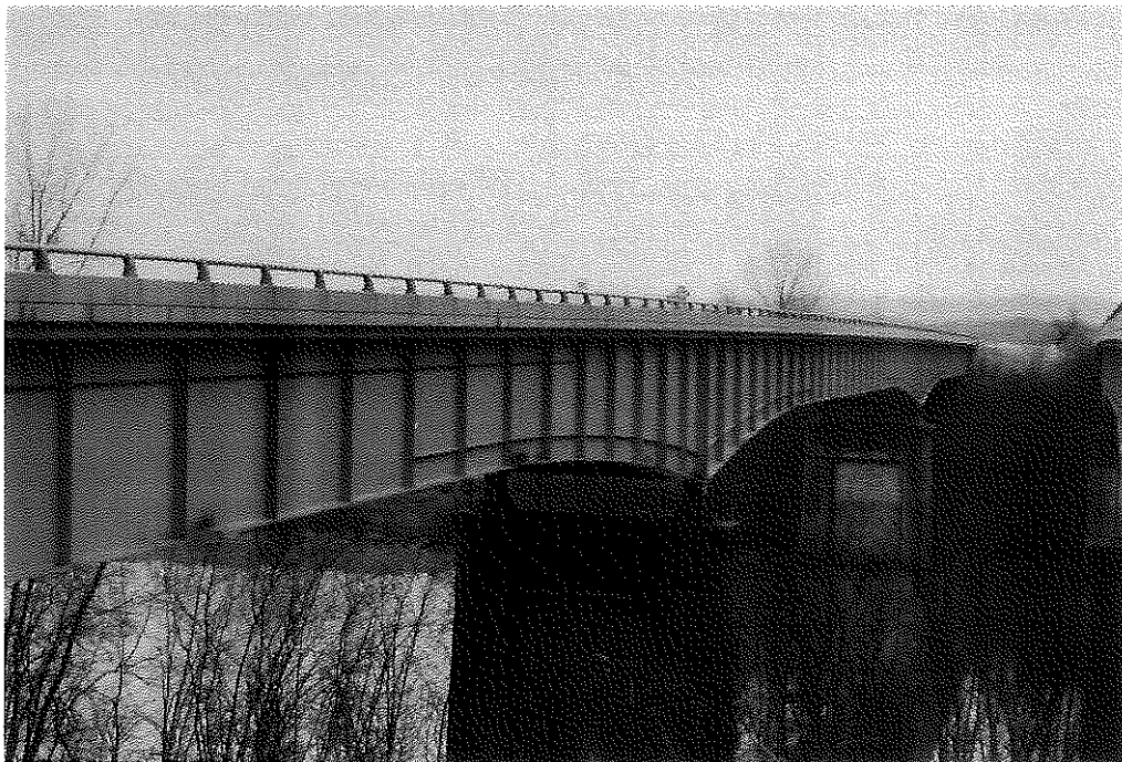
FIGURE 36. I-71 SOUTHBOUND MAINLINE BRIDGE OVER THE KENTUCKY RIVER SHOWING CORROSION ON LOWER WEB AND FLANGE. NOTE THE CORROSION UNDER DECK JOINTS (1997).
