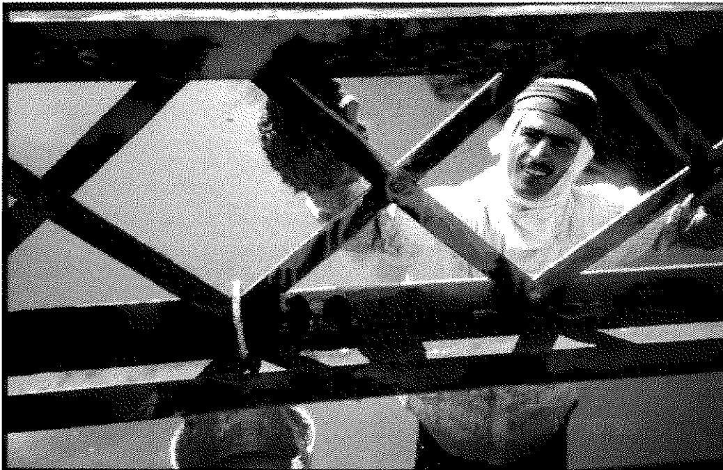
FIGURE 5. PRESSURE WASHING OF THE I-71 NORTHBOUND BRIDGE OVER THE KENTUCKY RIVER AT CARROLTON. NOTE THE REMOVAL OF CHALK BY THE WASHING PROCESS.
