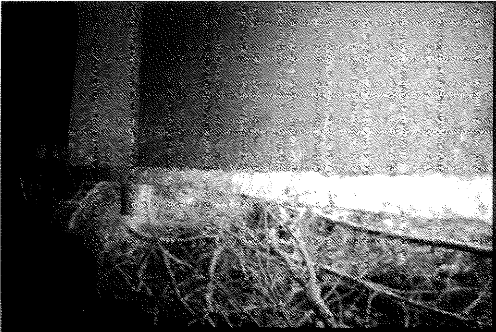
FIGURE 28. I-64 EASTBOUND OVER KY 420 SHOWING CORROSION WHERE COATING WAS APPLIED STRATIFIED RUST (1997).
