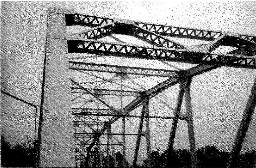
FIGURE 56. SOUTH SPAN END BENT, PORTAL AND UPPER CHORD OF KY 22 BRIDGE SHOWING PAINT IN GOOD CONDITION.
